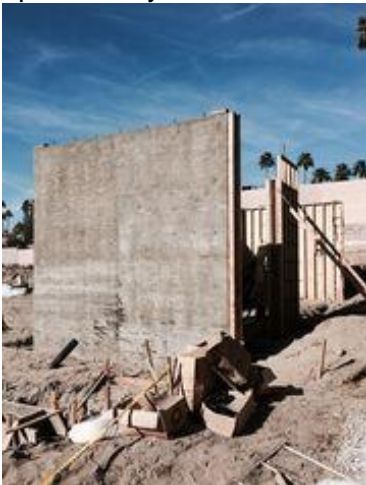
Poured concrete walls are beginning to take shape at site of the Arrive Palm Springs, the city's newest hotel construction, built from the ground up, in at least 10 years. (Photo: Submitted Photo: Chris Pardo)
