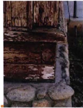
VERTICAL RAILROAD TIES WITH BATTEN & BOARD ABOVE SHAPED WATER TABLE OVER HORIZONTAL RAILROAD TIE
