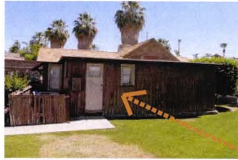
SOUTH FACING ELEVATION CONSTRUCTION ADDED 19XX. LANDSCAPE & IRRIGATION SHOULD BE REMOVED TO DECELERATE DETERIORATION AND TO NOT DAMAGE REPAIRED WALLS.
