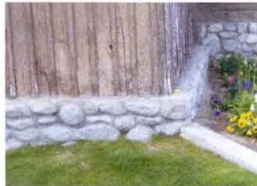
WATER DAMAGE TO VERTICAL BOARD & BATTEN AND INTERNAL WATER DAMAGE TO HORIZONTAL STACKED RAILROAD TIES
