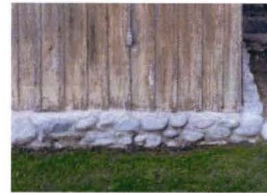
WATER DAMAGE TO VERTICAL BOARD & BATTEN
