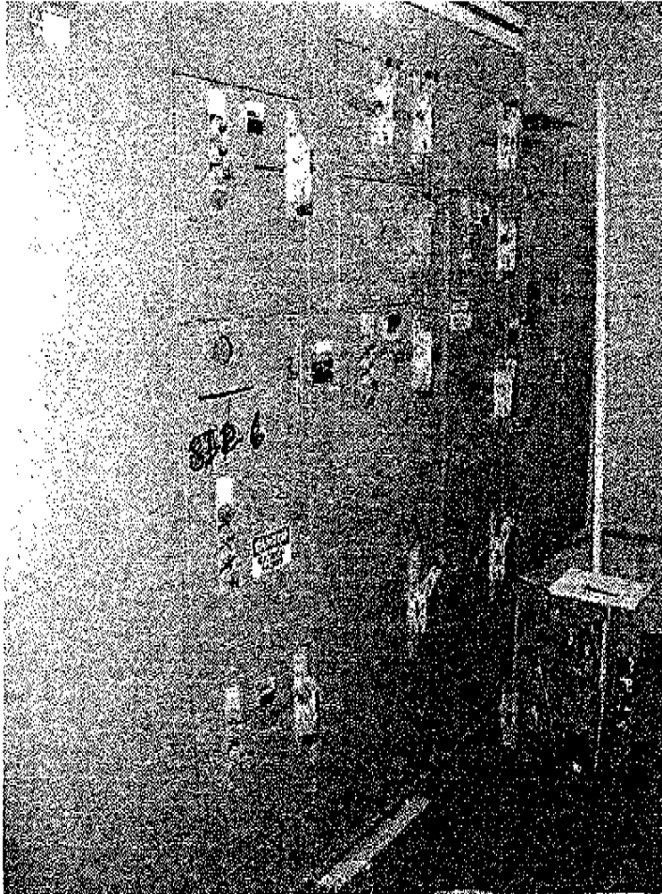
Figure 8 – Motor Control Center “#1MCC” at Maintenance Building
