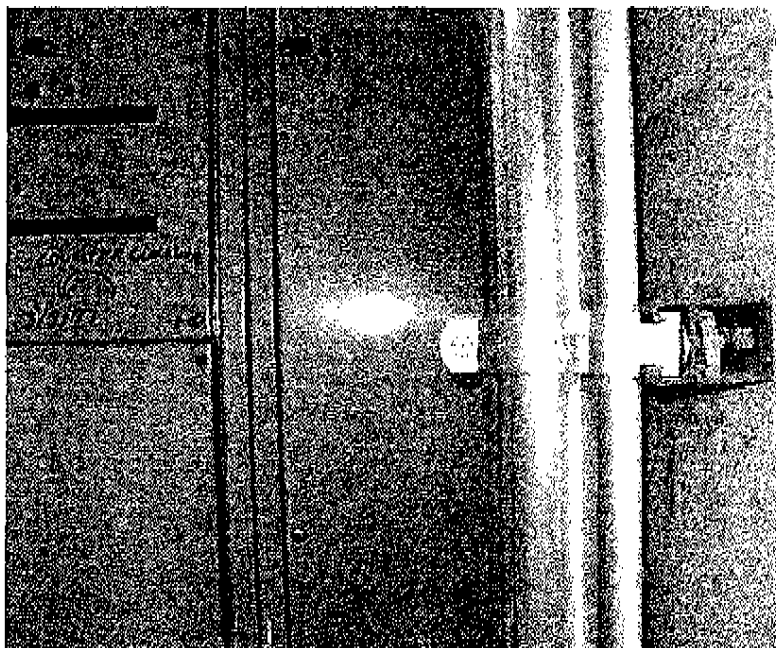
Figure 2 – Switchboard Front Access Interference in Administration Bldg.
