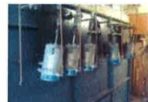
Pneumatic Controls on Multi-zone-AHU
