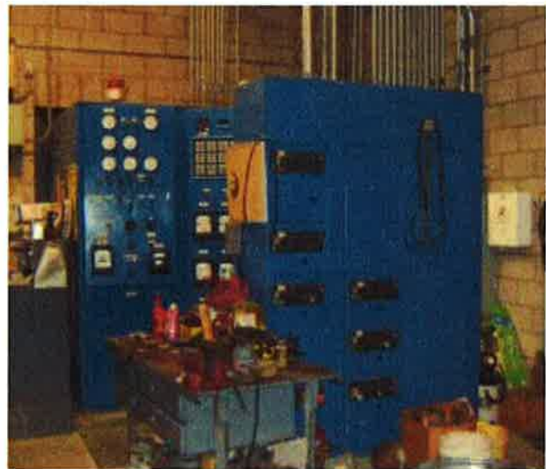
Synchronizing Switchgear and MCC
