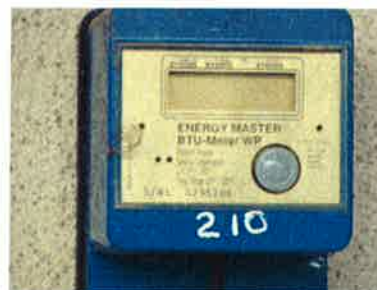
Existing BTU-Meter not Working
