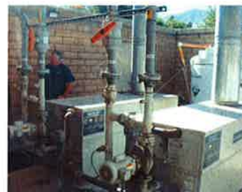
Swimming Pool Boilers
