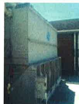
BAC Cooling Tower
