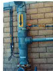
Cogeneration HHW Supplementing Pool Heating
