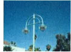
Exterior Lighting Fixture
