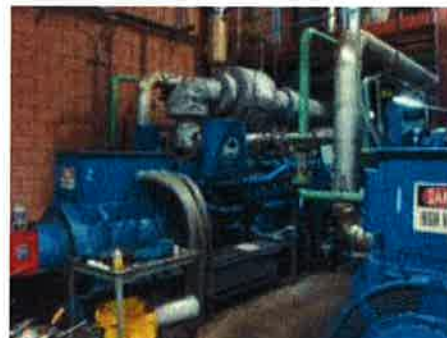
Caterpillar Engine Generator(s)
