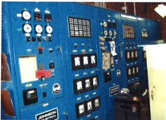
Synchronizing Switchgear and MCC
