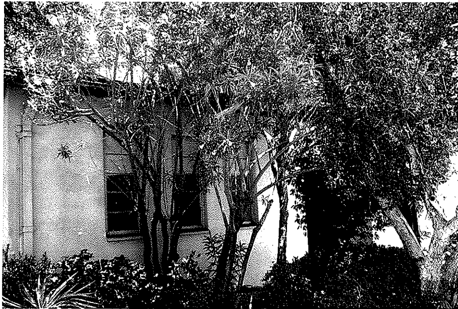
Trees and Shrubs Against Building
