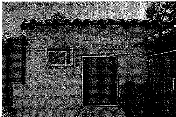
A/C Units and Exposed Conduit
