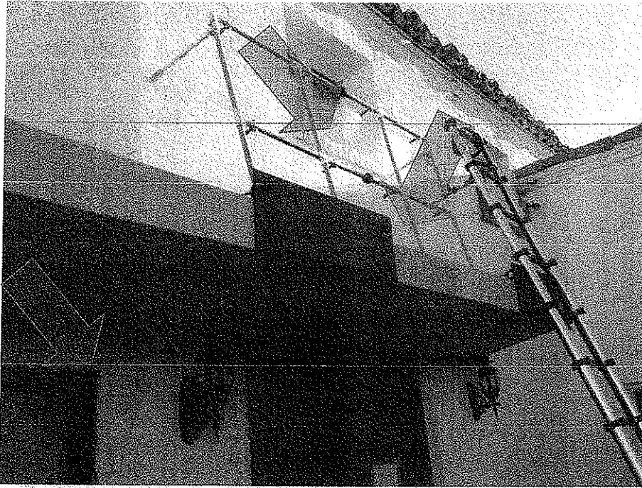
PHOTO 9 – Water test above the entry door of the restaurant produced a leak into the dining room below. The window above the entry door also leak at the window frame. The wall above the entry door also leaked – see blue arrows.
