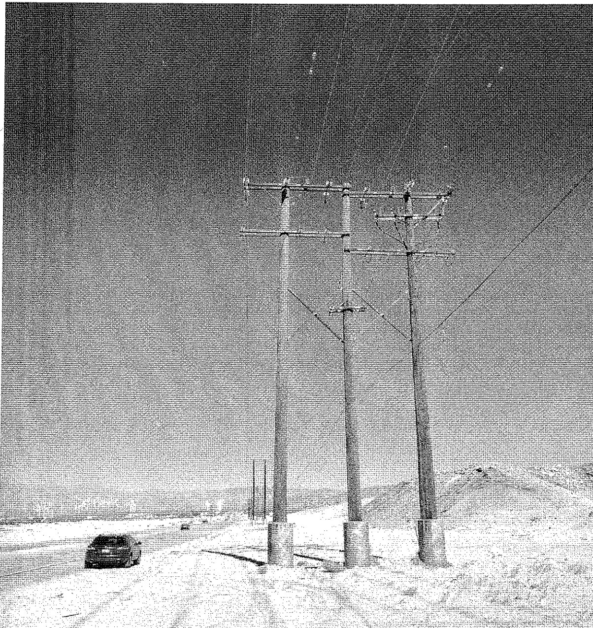
Large Structure just south of property Large Structures with 2x33kv; 2x13kv; and telecom line – designated for removal
