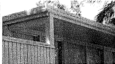
CURRENT CONDITION WITH TRIM STRIP
