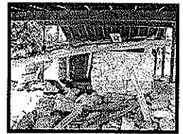
Collapsed east wall of the Old Adobe
