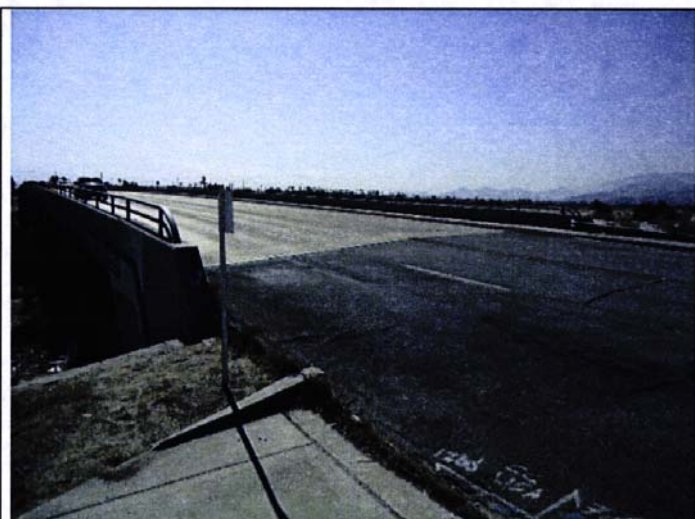
Photo No. 5 – Southeast view of Ramon Road from western part of bridge.
