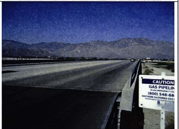
Photo No. 4 – West view of Ramon Road from eastern part of bridge.
