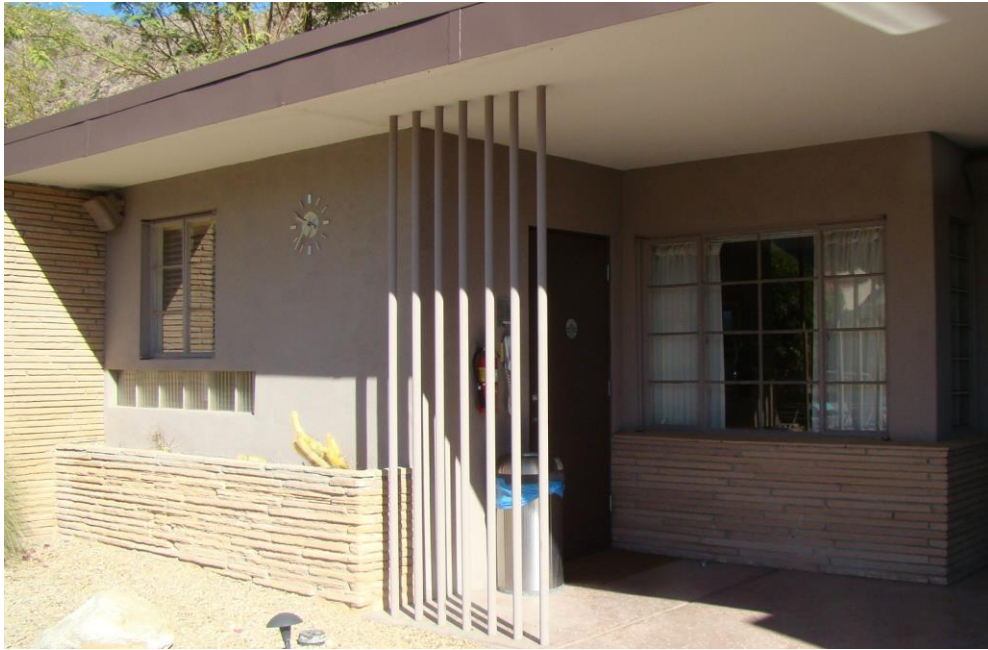
Detail of mortared stacked sandstone planter (left), stacked sandstone pier (far left), stacked sandstone wainscoting (right), metal pipe supports (center), casement windows and glass block
