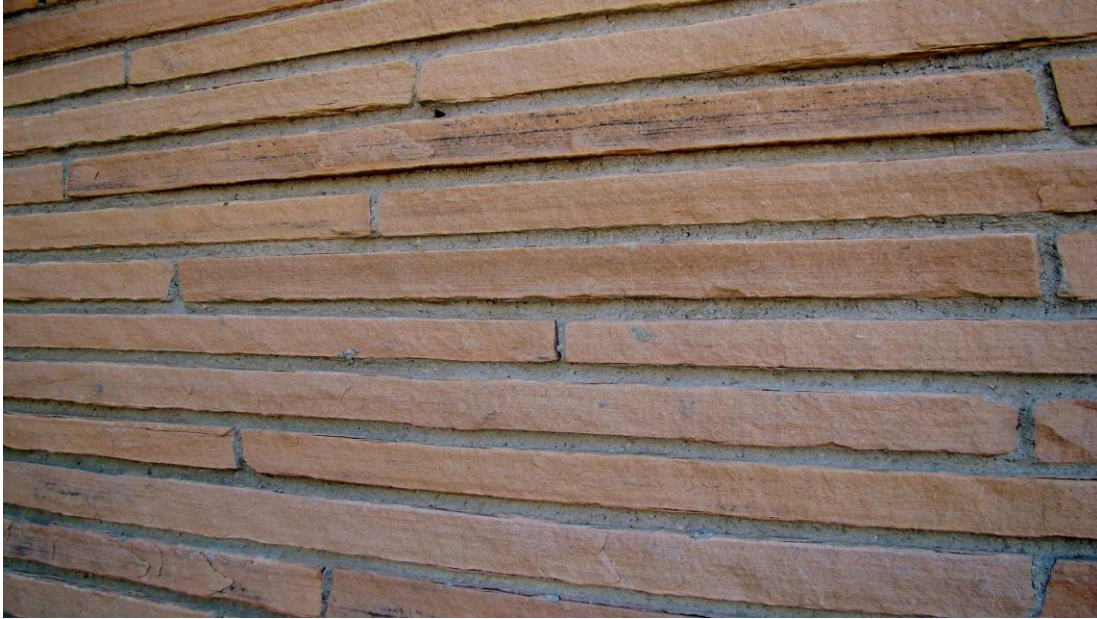
Detail of mortared stacked sandstone laid ledge-style. The length of these sandstone slabs can vary from 4 inches to almost 36 inches
