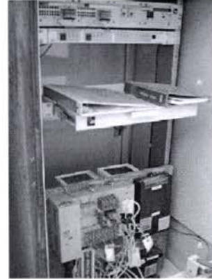
EXISTING TELCO BOX
