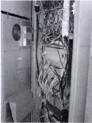
POWER FROM MM-BTS CABINET
