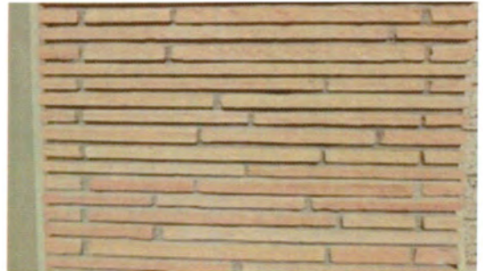
Photo by Clara Nelson Detail of original mortared and stacked flagstone pier
