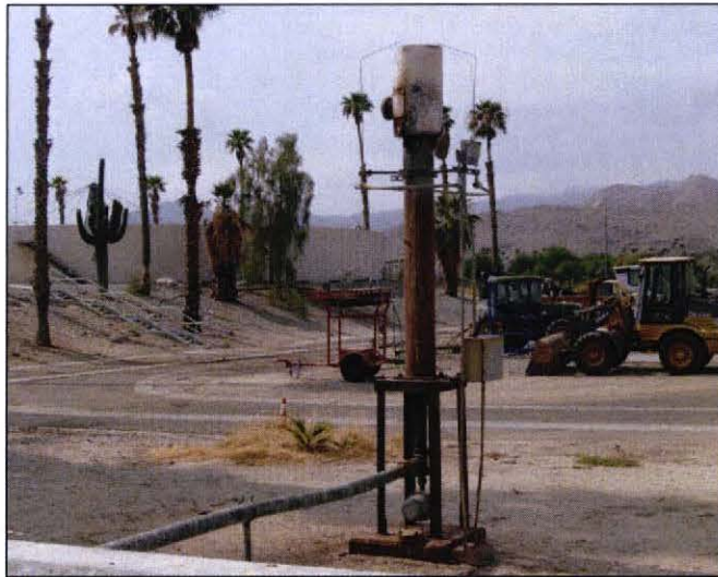
Photo of the Digester Gas Flare
