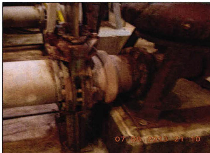
Photo of Lift Station No. 1 Pumps and Valves
