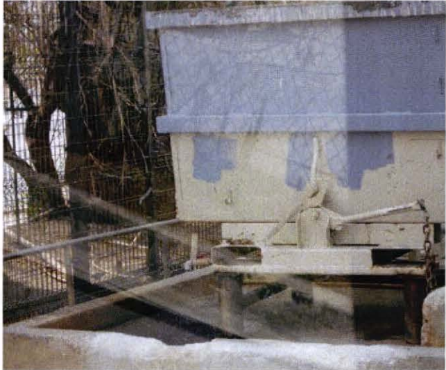
Photo of Damage to Concrete Containment
