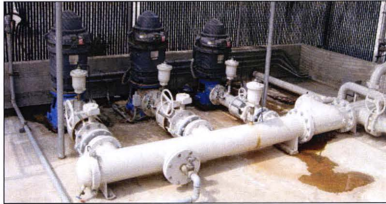
Photo of Standing Water at Recycled Water Pump Station
