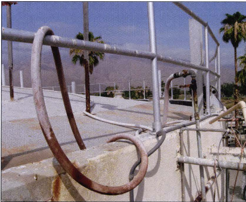
Photos of Corrosion on Anaerobic Digester No. 1 Cover
