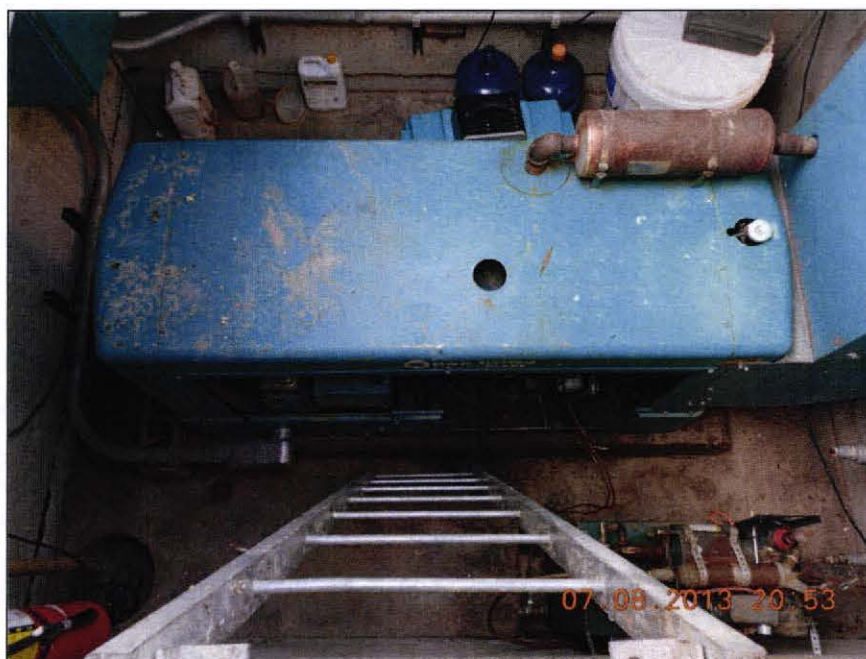
Photo of Emergency Generator at Lift Station No. 4
