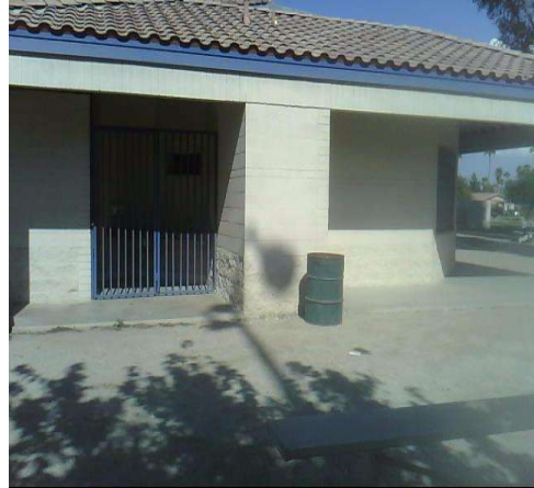
Path Of Travel , Walking Surfaces : Noncompliant Surface
