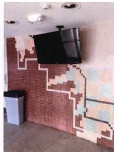
EXISTING LOBBY VIDEO MONITOR
