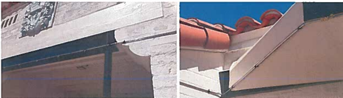
DETAIL ABOVE THE PASEO LEADING TO PALM CANYON AND AT NORTHWEST CORNER SHOWING NEW MISTING PIPING
