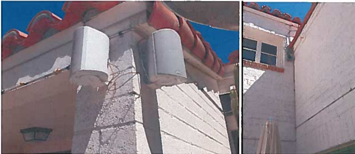
DETAIL ALONG THE NORTH WALL OF THE COURTYARD AND THE NORTHEAST CORNER SHOWING NEW MISTING PIPING
