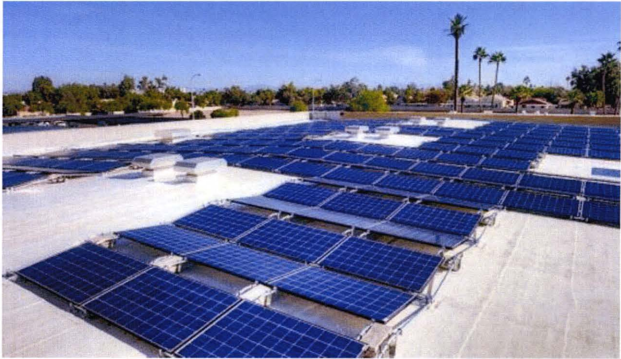
Figure 3 Convention Center Solar PV System
