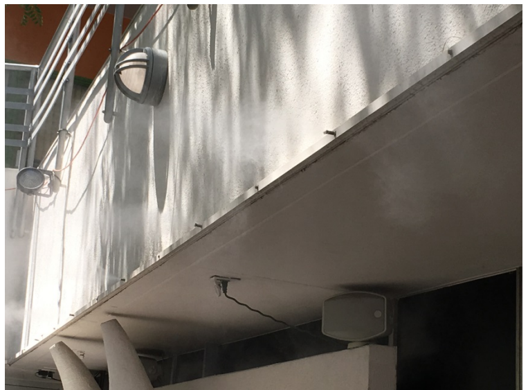
Misters at the Oasis building
