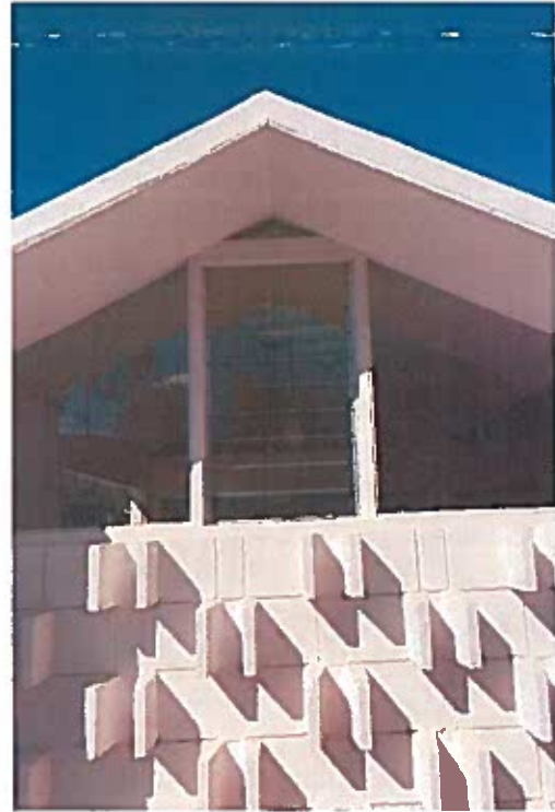
Non-Conforming Clerestory Window
