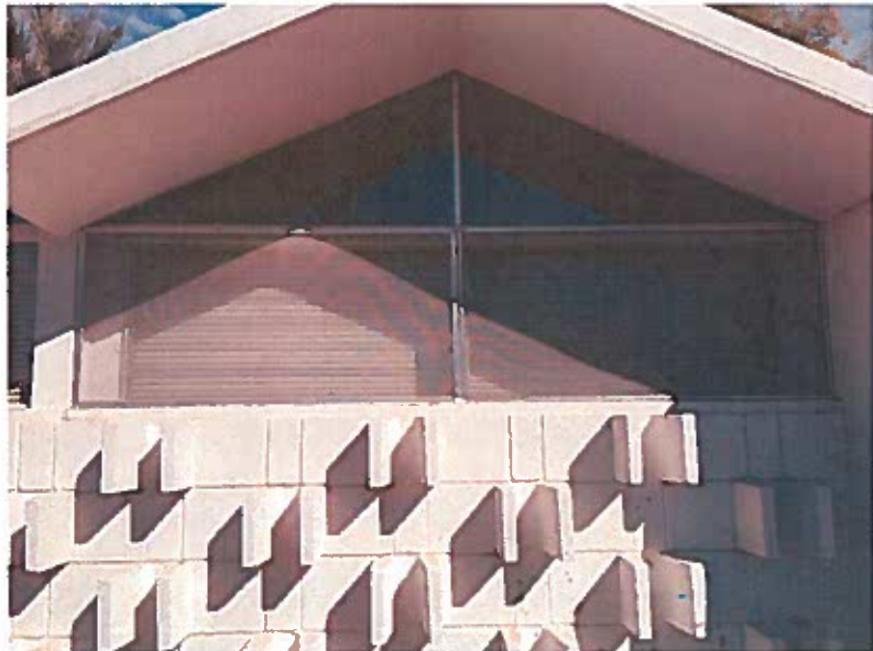
Non-conforming Clerestory Window
