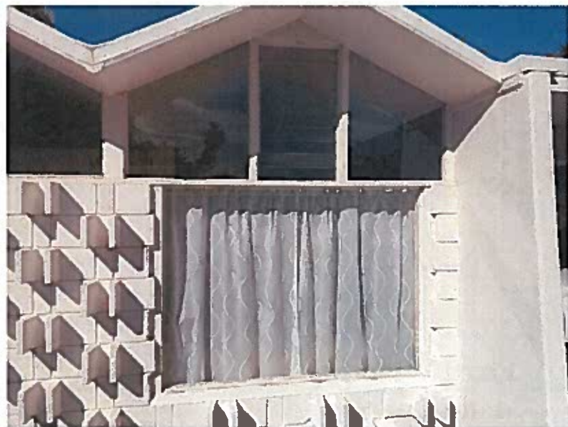
Block Removed Non-conforming Clerestory Window
