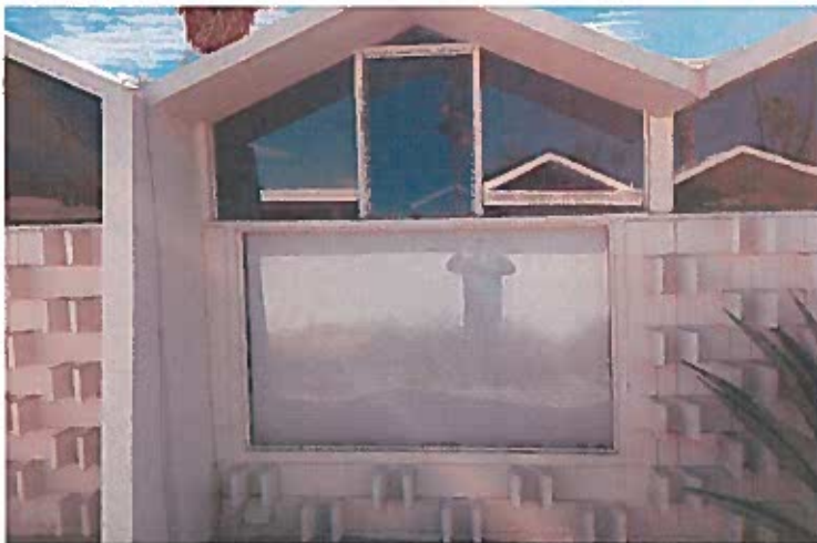
Block Removed Non-conforming Clerestory Window
