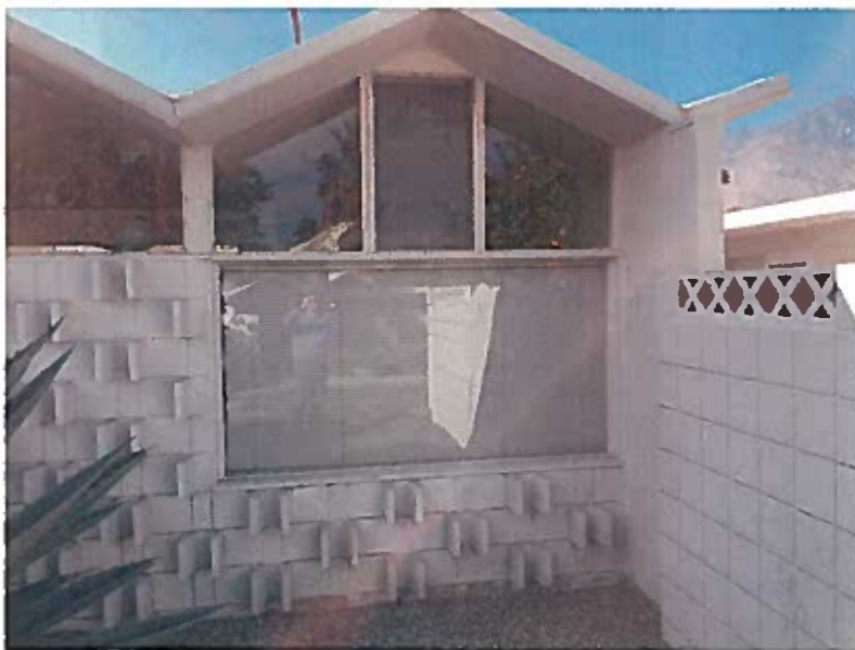
Block Removed Non-conforming Clerestory Window
