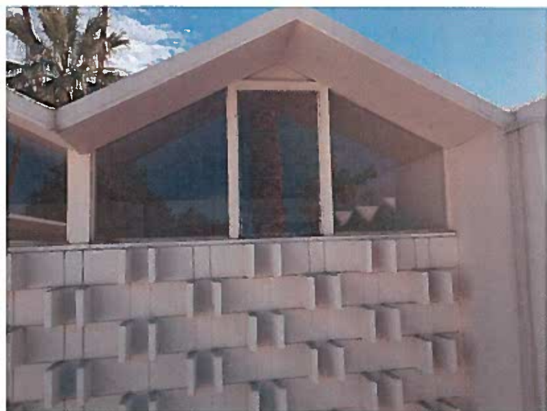
Non-conforming Clerestory Window
