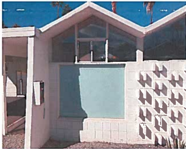
Block Removed Non-conforming Clerestory Window
