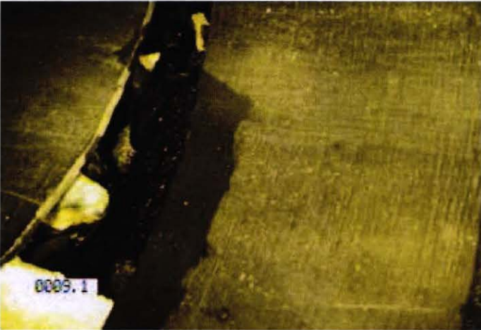
CC - Crack Circumferential @ 9.1 ft.
