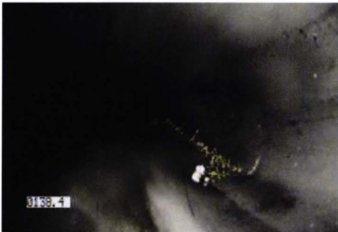
D - Pipe Deformed @ 138.4 ft.
