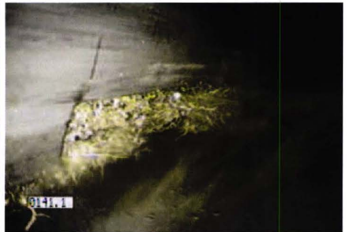
BSV - Pipe Broken: Soil Visible @ 141.1 ft.
