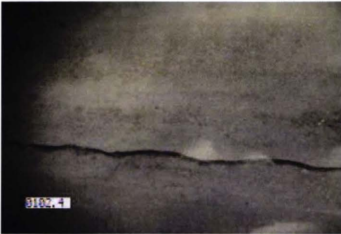
CL - Crack Longitudinal @ 102.4 ft.
