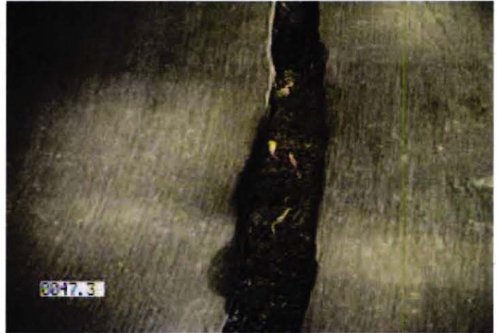
CC - Crack Circumferential @ 47.3 ft.
