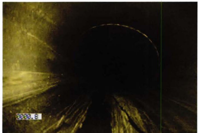
D - Pipe Deformed @ 0.8 ft.
