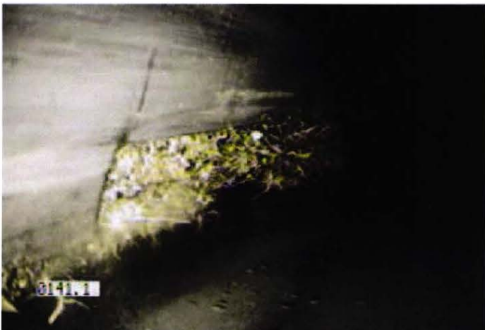
BSV - Pipe Broken: Soil Visible @ 141.1 ft. pipe broken roots
