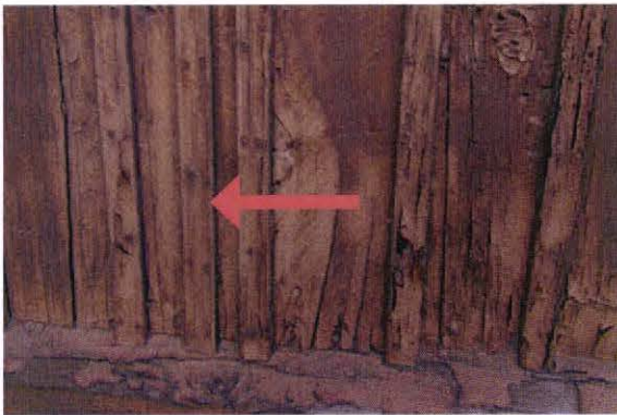
Cross ties and battens at east elevation. Note additional batten at left of image
