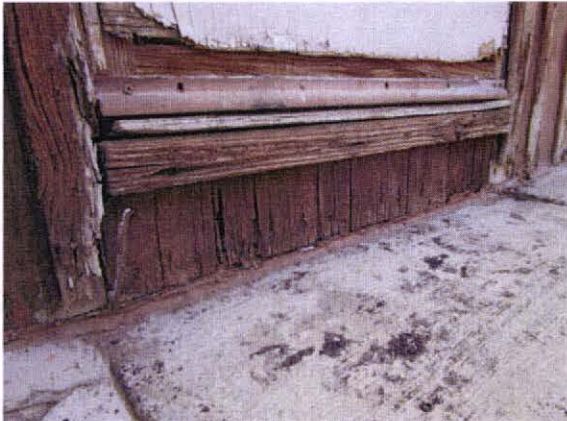
Decay at base of Kitchen door.
