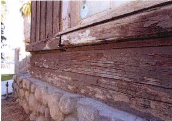
Heavy decay at cross ties at west elevation.
