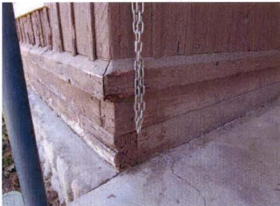
Typical view of paint coatings. Note relatively intact paint layer at protected porch (right) side and deteriorated layer at exterior (left) side.
