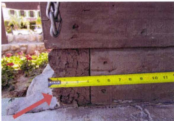
Decay and section loss at cross tie at northwest corner of Bathroom.
