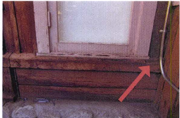
Belt course at south elevation of Dining Room. Note notch at right side.
