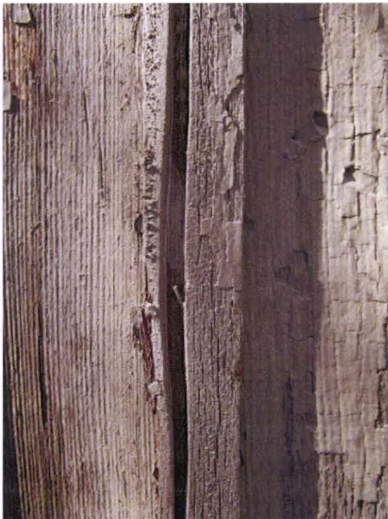
Split batten at east elevation.
