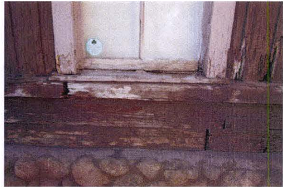
Heavy decay at belt course at west elevation.
