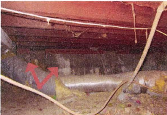
View inside crawlspace to west foundation wall below Kitchen. Note engaged piers and blocking with stone between.
