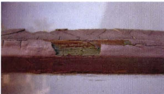
Detail view of window muntin at west elevation. Note mint green paint.
