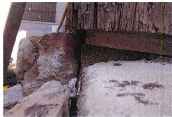
Detail view of concrete slab. Note proximity of concrete and stone to wood framing.
