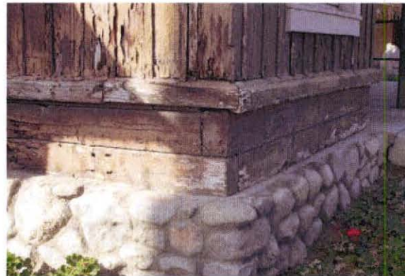
Heavy decay at cross ties at northeast corner.
