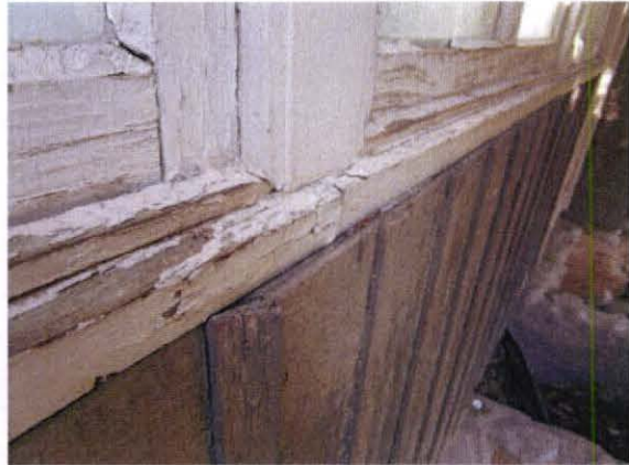
Displaced siding at east elevation of Second Room.
