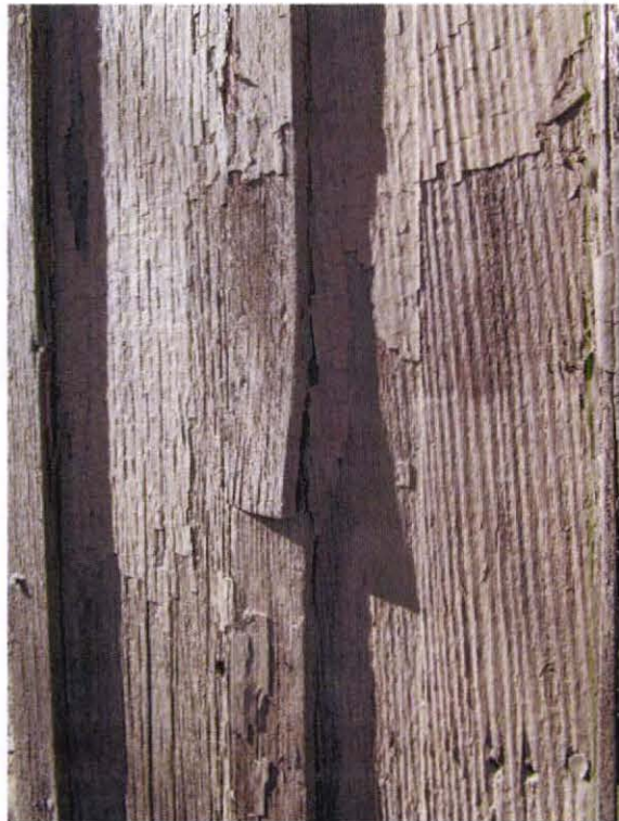
Warped batten at east elevation.
