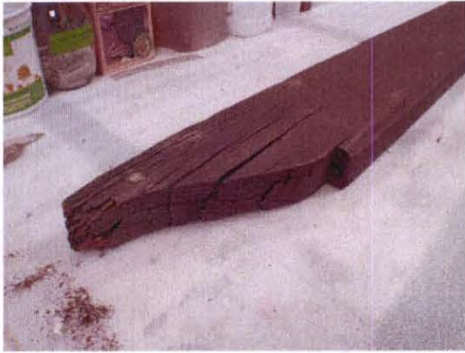
1. Rafter prior to treatment.
