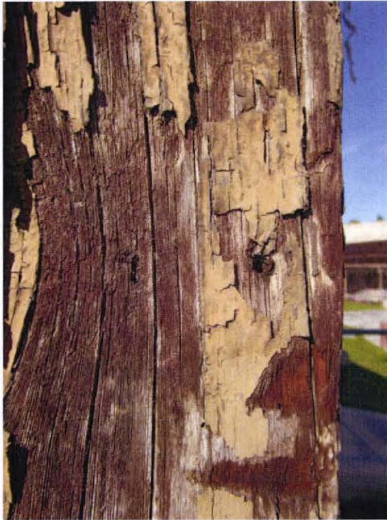
Detail view of heavily deteriorated paint. Note white residue which could be old primer or paint layer.
