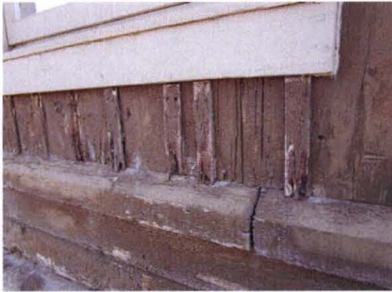
Decayed, missing and added battens at north elevation.
