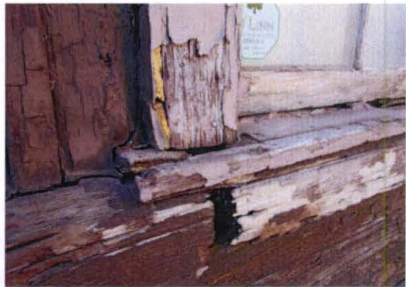
Advanced decay at Dining Room window at west elevation.
