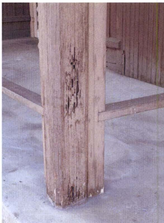
View of decay at porch column and base of balustrade post.
