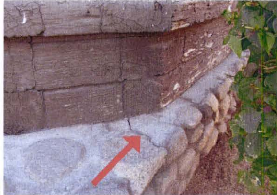
Concrete and stone foundation wall at northwest chamfered corner. Note crack in wall.
