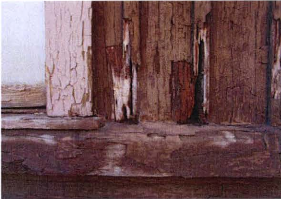
Heavy decay at base of cross ties above belt course at west elevation.
