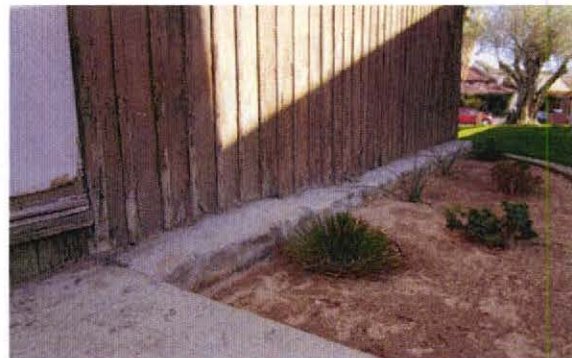
Rise at foundation wall, south elevation.
