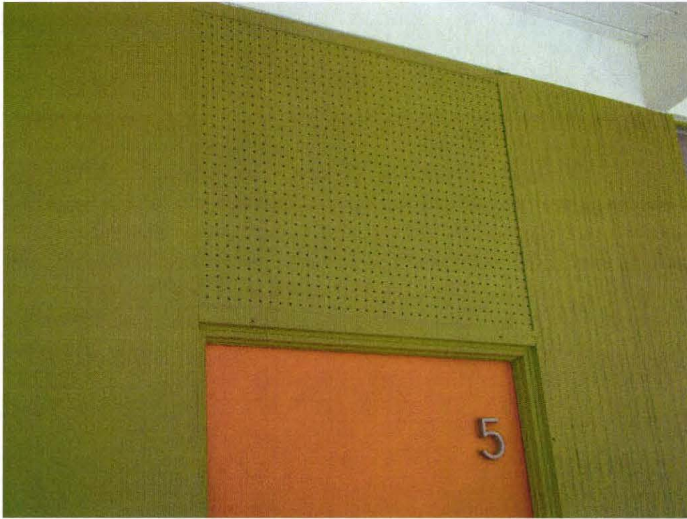
This decorative pegboard insert above the door serves to emphasize the verticality of the door and echoes the use of the material in the light sconce.
