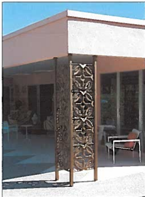
Steel 2"x2" support columns and AGUs.
