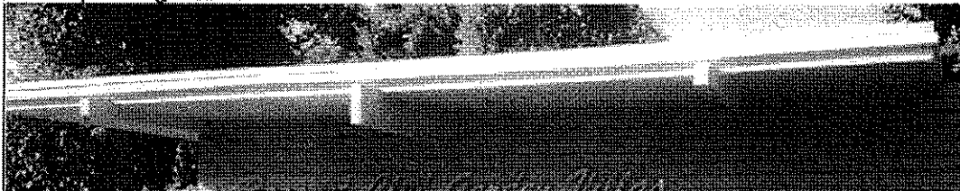
THIS MOTIF OF "SHORT-DEEP-SHORT" CANTILEVERED BEAMS OCCURS IN NUMEROUS LOCATIONS THROUGHOUT THE DISTRICT
