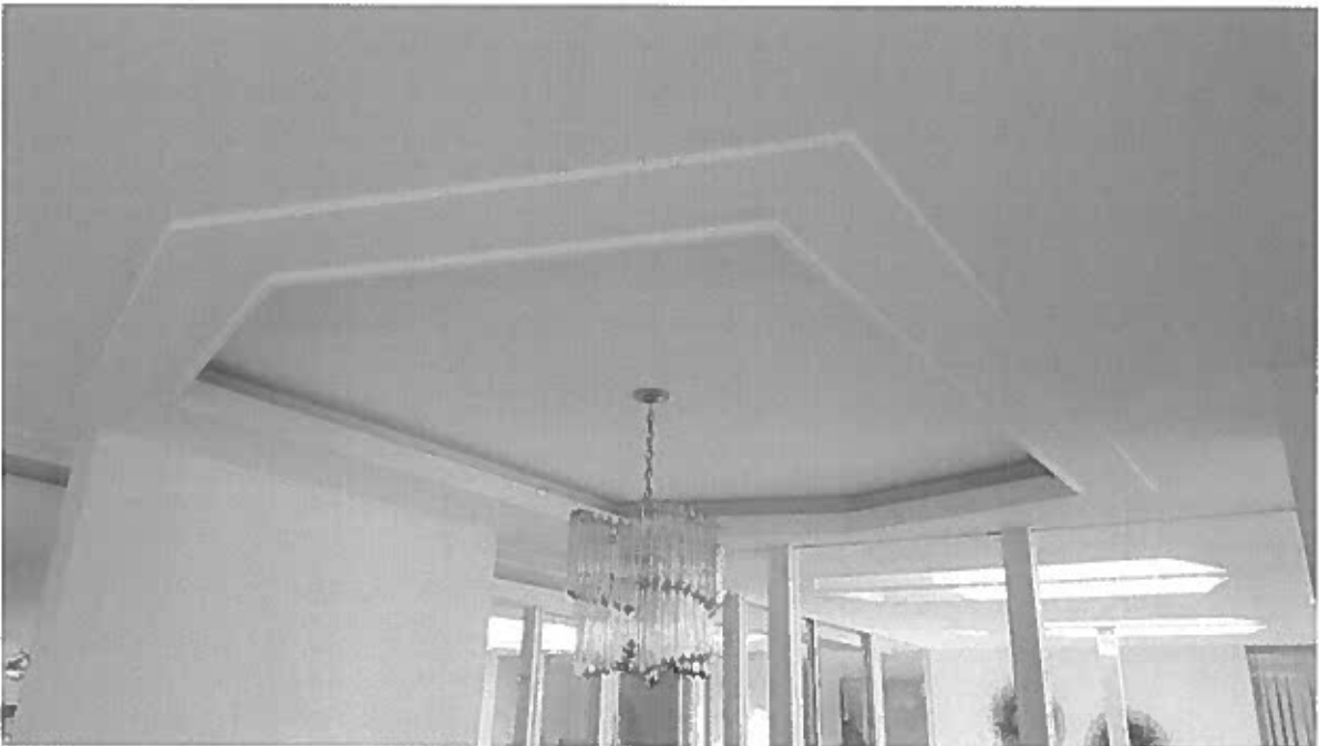
Tray ceiling over dining area. Tray ceilings can also be found in the main hallway.
