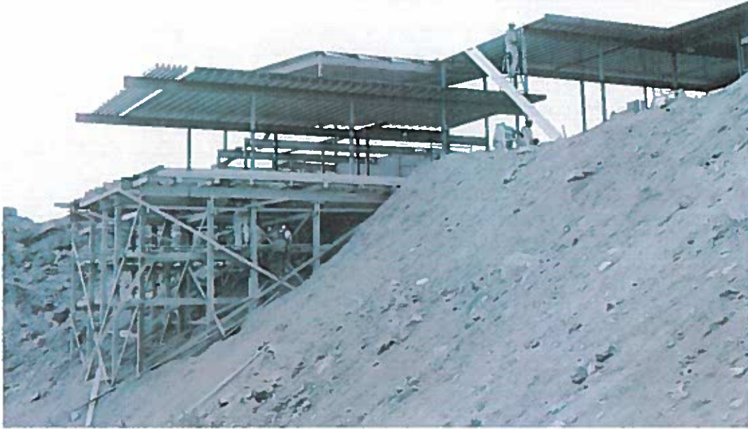
Construction of cantilevered living room volume. Hugh Kaptur Collection, Palm Springs Art Museum.
