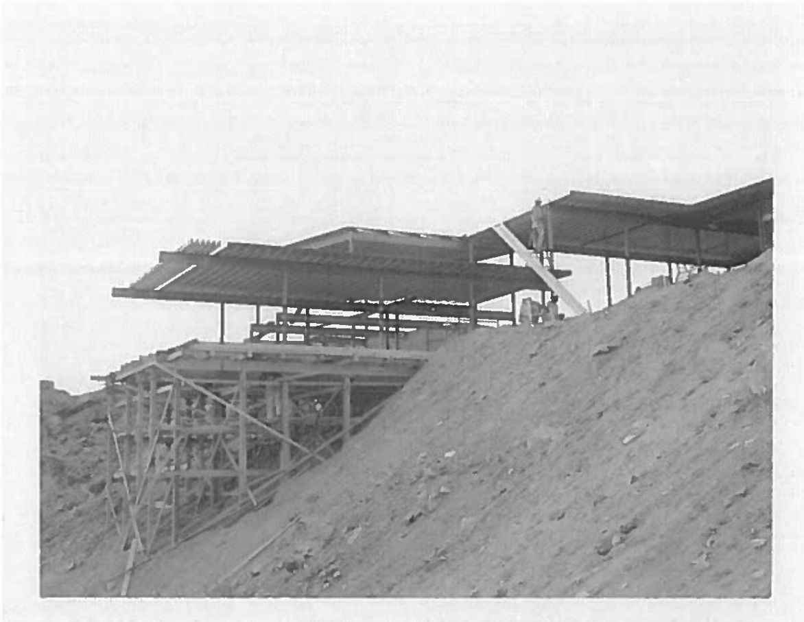
Construction of cantilevered living room volume. Hugh Kaptur Collection, Palm Springs Art Museum.
