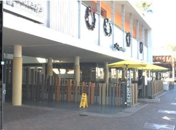
BELOW RIGHT: THE OPEN FEELING OF THE FIRST FLOOR PLAZA HAS BEEN ADVERSELY AFFECTED BY FENCES AND BARRIERS.
