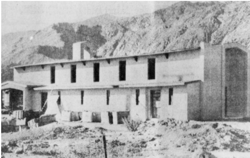
Our Lady of Guadalupe church under construction in December of 1963. Source: The Desert Sun , December 13, 1963.
