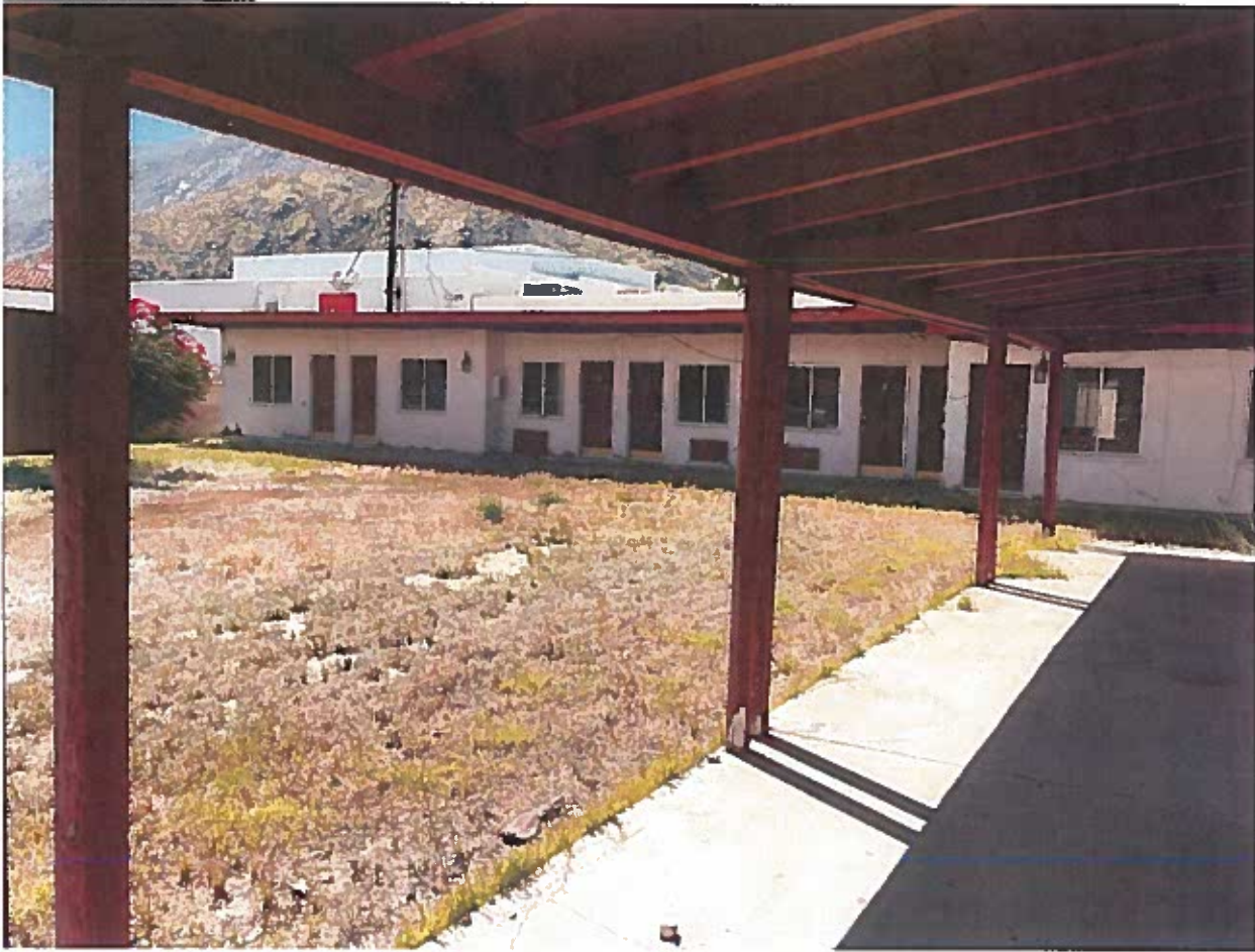
Photo 8: Crawford Apartments: Building "B" south portion in background, Building "A" covered porch in the foreground.
