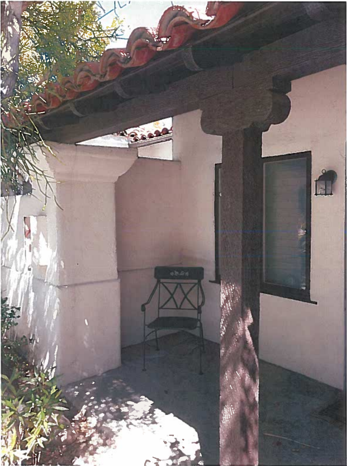
Photo 41 Harlow Haven Bldg D west elevation typical covered front porch wood rafter tails, detail at top of wood post and corbelled stucco pilaster
