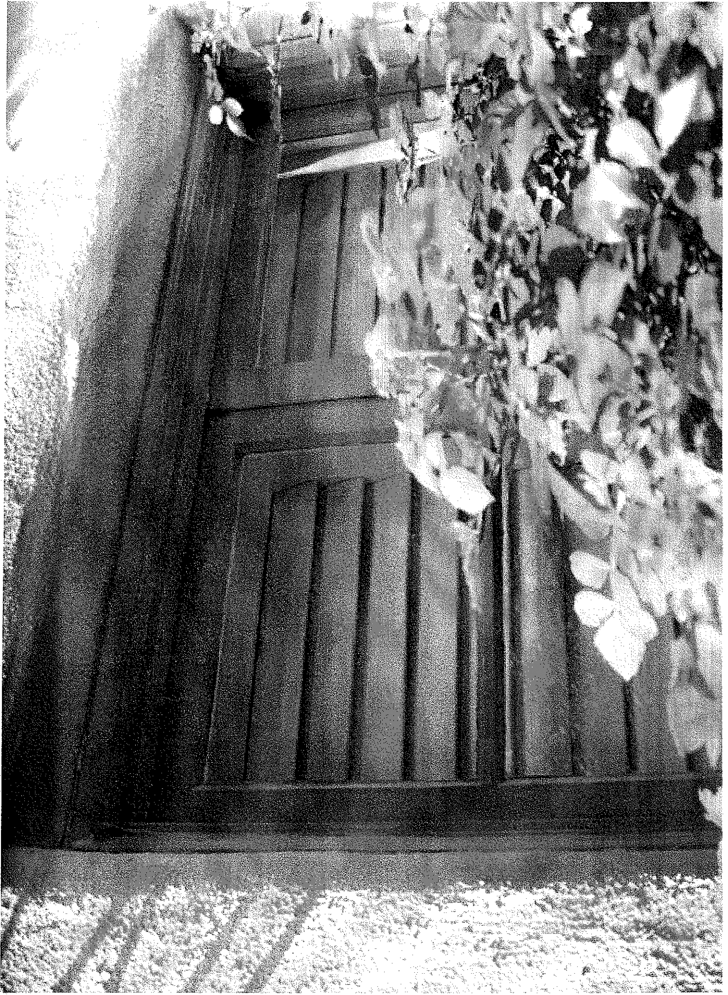
PHOTO 5 - B: Original window framing. Located on the North side of the house.
