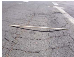
Rutting and Depressions
