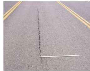
Longitudinal and Transverse Cracking
