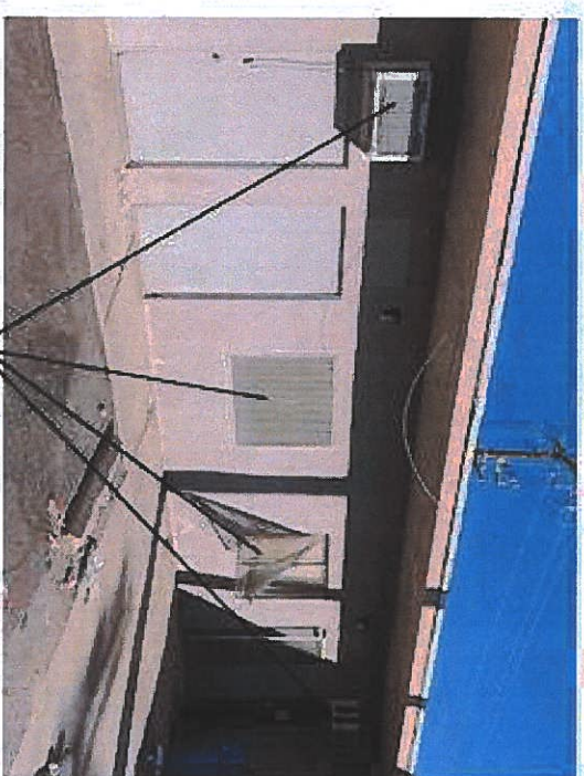
Remove and repair all mismatched doors, screens, and windows. Remove A/C wall unit
