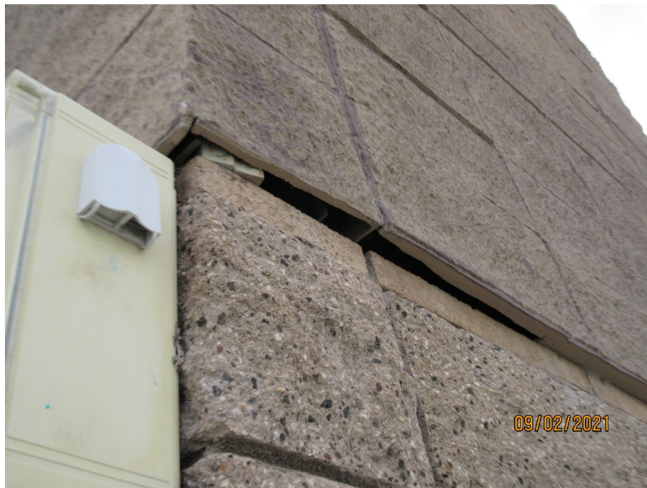
Faux block material on existing Verizon facility
