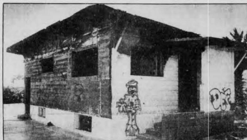
SIGNS OF DETERIORATION . . . are evident in Palm Springs' predominantly black neighborhoods. A fire-gutted house which now attracts only vandals and graffiti
