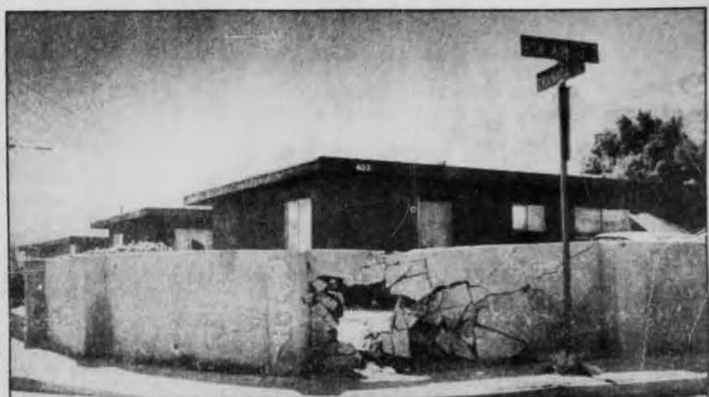
and a crumbling wall are graphic testimony of the problems which residents say still exist for black people in Palm Springs.
