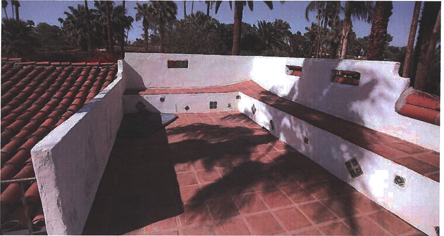
37 view north of roofdeck; note unsafe railings and awkward construction at northeast corner suggestion this was an addition that was not well integrated with existing construction
