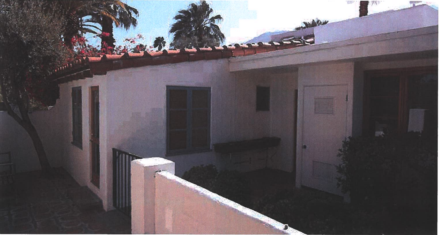
14 view southwest from backyard toward bedroom 5 (left) and kitchen (right); note the different roofline of bedroom and kitchen
