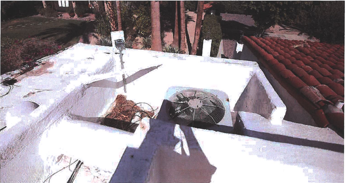
35 view northeast from roof deck over kitchen roof; note mechanical equipment and poor drainage
