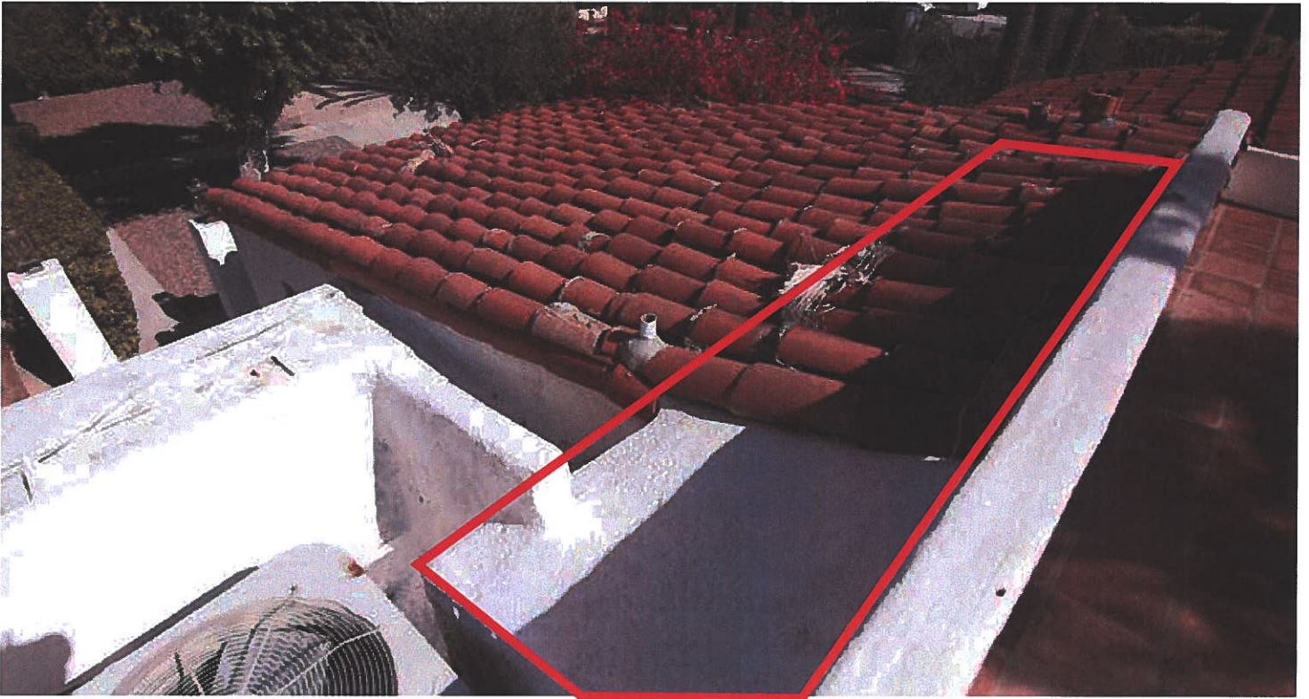
33 view southeast from roofdeck over bedroom 5 roof; red highlighted area was an exterior space at one time and was enclosed to create a mechanical room
