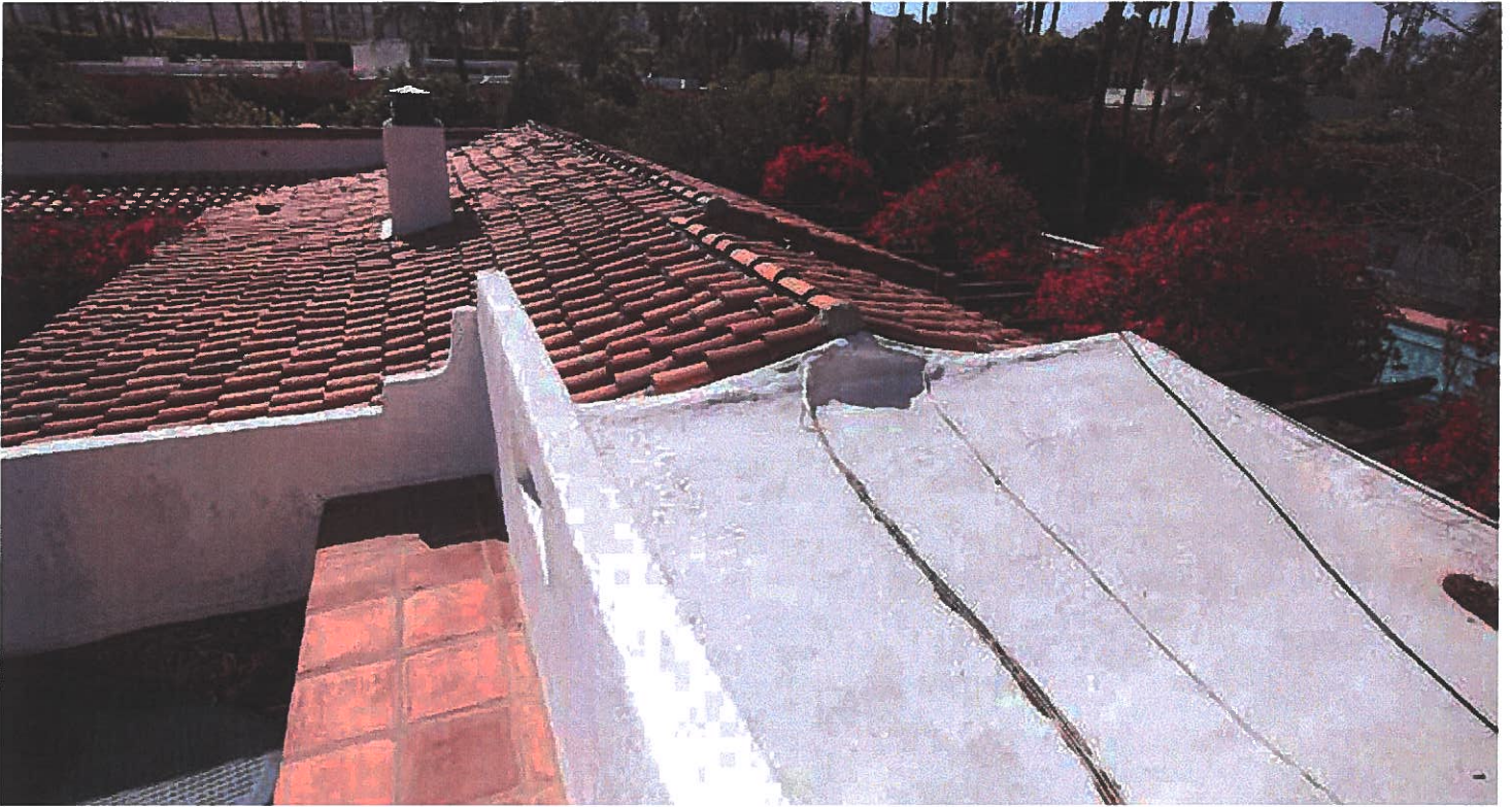
31 view west from roof deck across living room roof with kitchen roof on right (white BUR)
