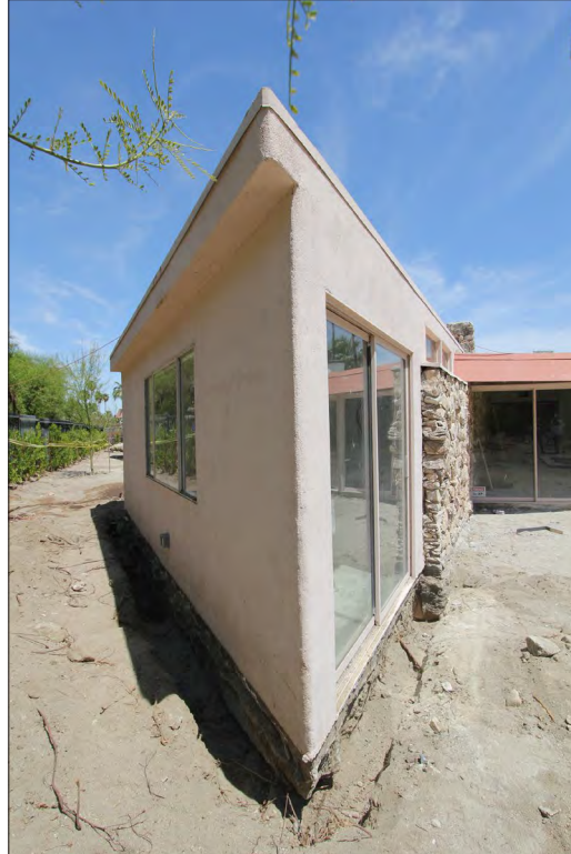
Image 32: Subject property, exterior, north (left) and west (right) elevations, room addition, view southeast (Chattel, 2021)
