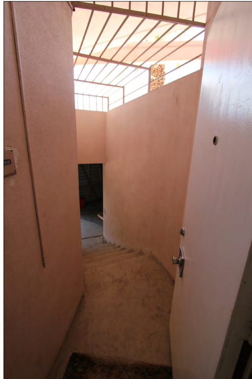
Image 76: Subject property, interior, stairs to carport, view east, note security bars shown in Image 44 (Chattel, 2021)
