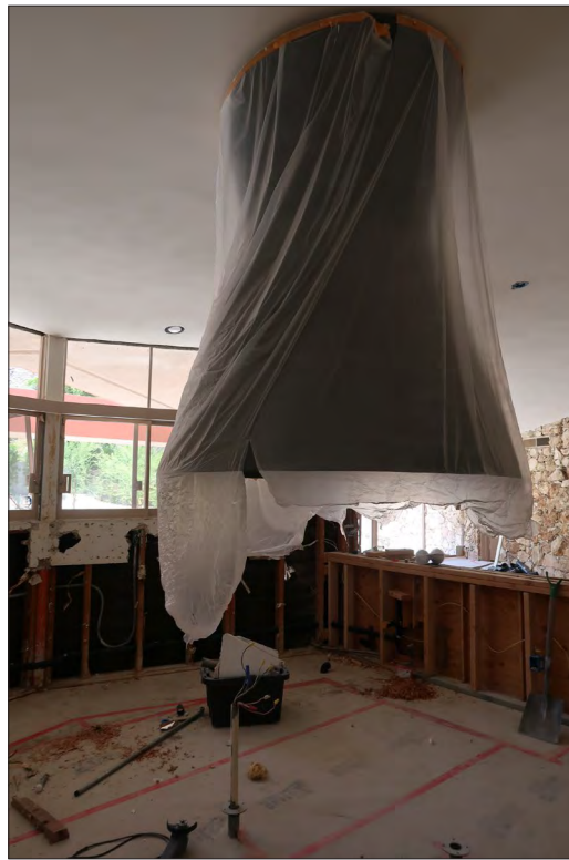
Image 55: Subject property, interior, kitchen, detail of conical sheet metal vent, view west (Chattel, 2021)
