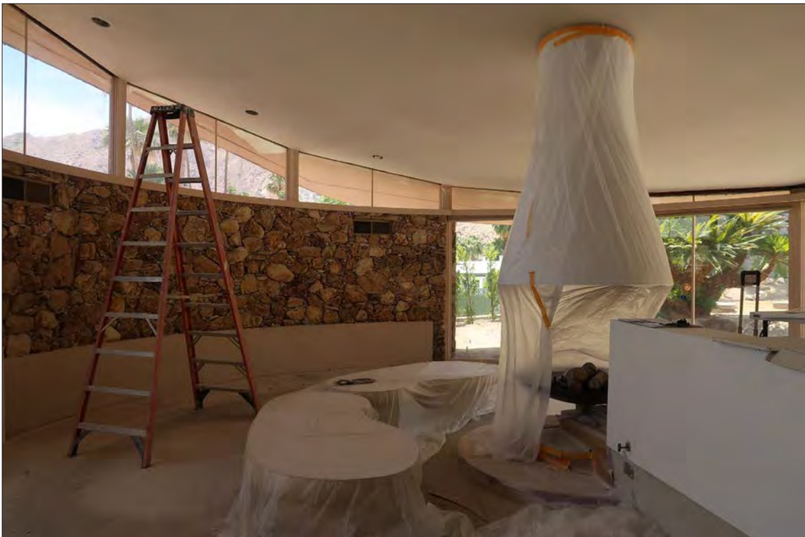
Image 50: Subject property, interior clad wall, clerestory windows, conical sheet metal vent, and low dividing wall (Chattel, 2021)
