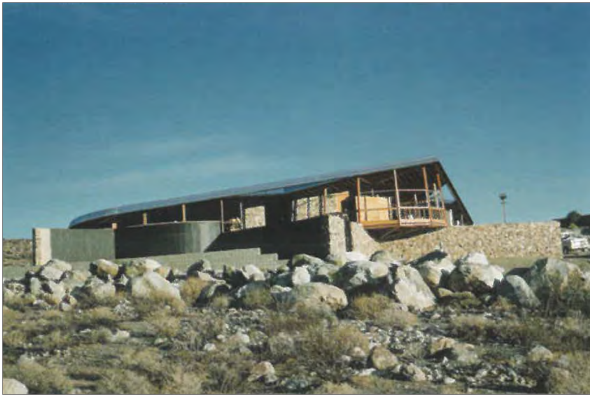
Image 2: Subject property under construction, view north (Harlan, The Alexanders: A Desert Legacy, Kitnick Family Collection, c. 1960)
