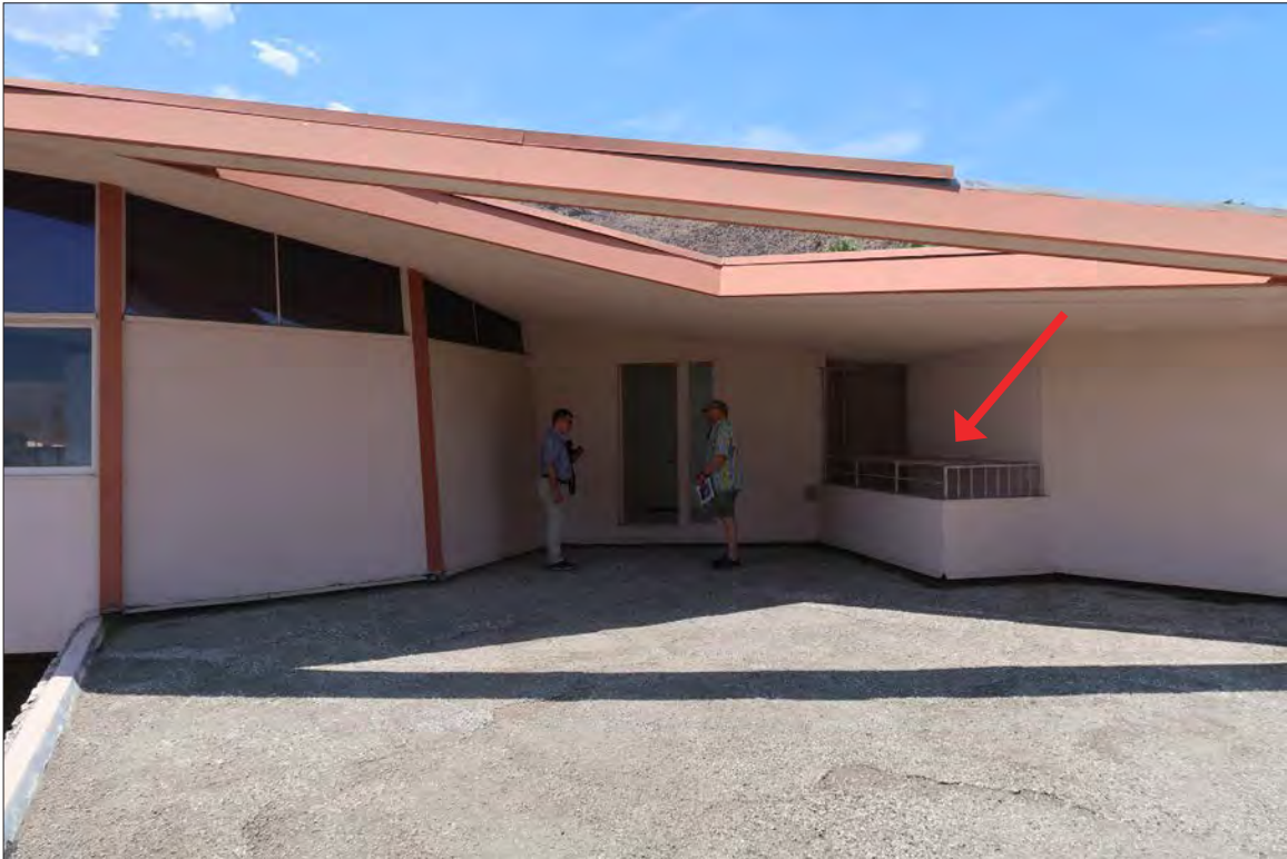
Image 44: Subject property, exterior, east elevation, roof of carport accessed via door in master bathroom, view west, note security bar above stairs to carport
