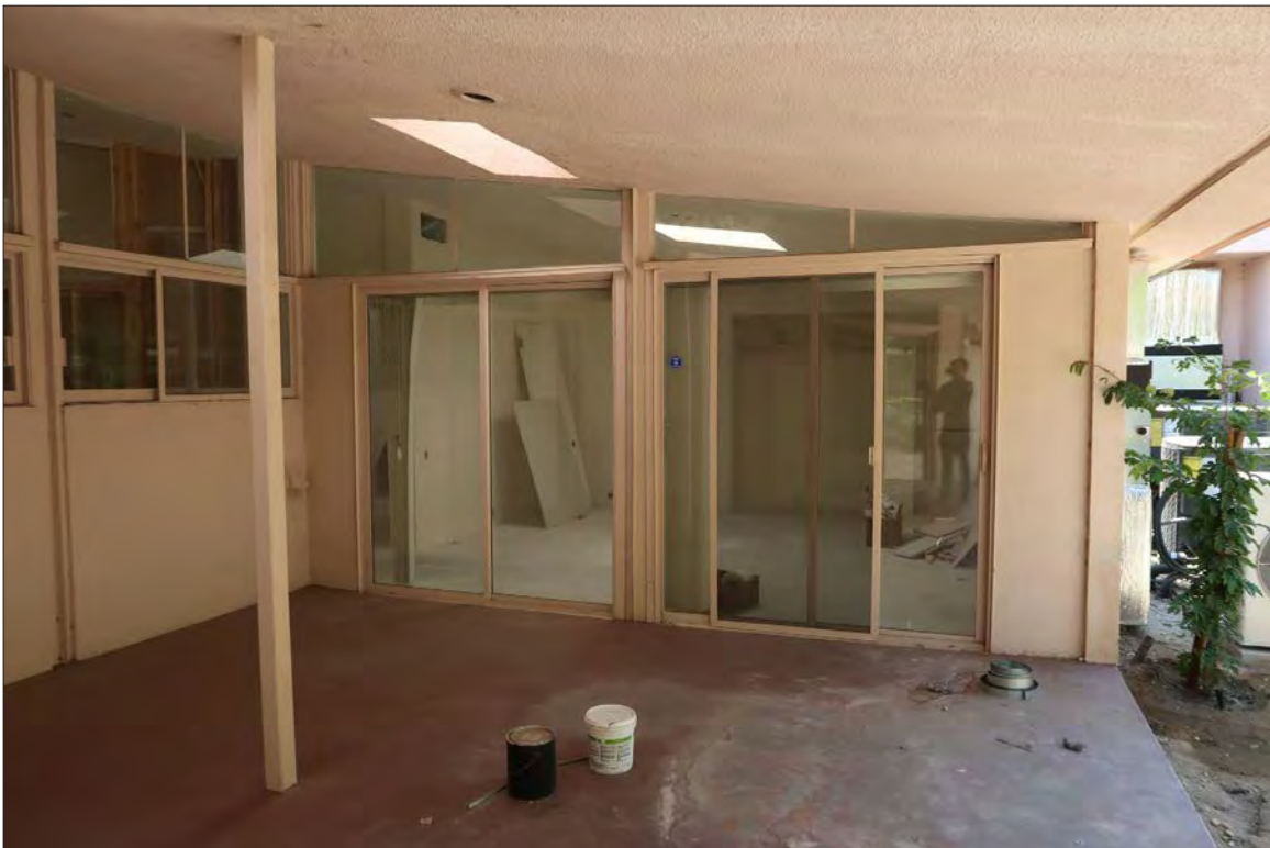
Image 24: Subject property, exterior, north elevation, sliding doors at inset patio, view southwest (Chattel, 2021)
