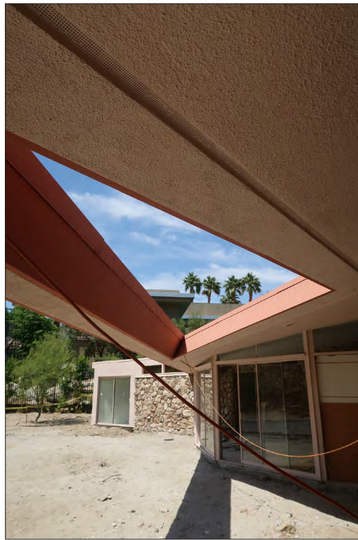
Image 37: Subject property, exterior, west elevation, detail of triangular cutout in roof, view north (Chattel, 2021)
