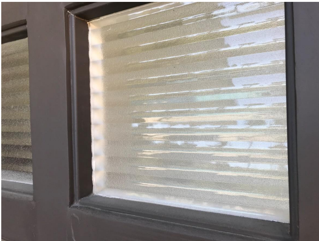
The restored box grid and obscure glass decorative wall. Each pane of glass had to be individually measured and cut, as the sizes varied. Author's photos.
