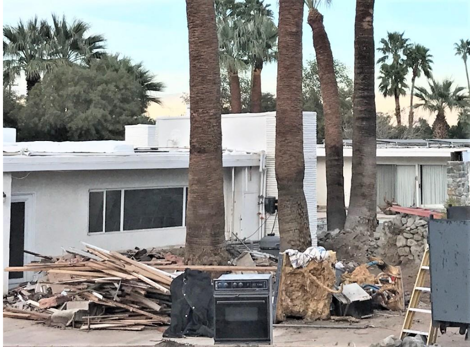
In this February 2019 photo, the Arizona sandstone planter had fallen into disrepair, with half of the sandstone missing. Also, unsightly pipes and wires had been installed over the years. Author's photo.
