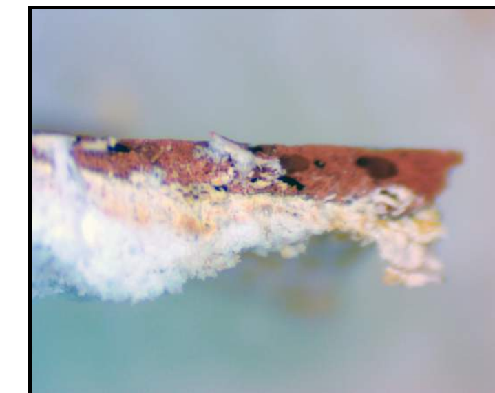
SAMPLE NO. 49 WALL FINISH AT SOUTH ATMOSPHERIC WALL AT UPPER WALL NEAR CENTER 5. MODERATE VERMILLION 4. YELLOWISH-WHITE/CREAM 3. LIGHT YELLOW OCHRE 2. MEDIUM YELLOW OCHRE 1. YELLOWISH-WHITE/CREAM
