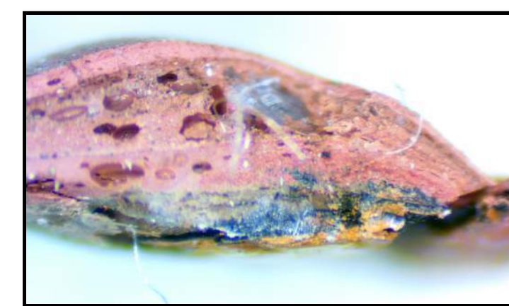
SAMPLE NO. 13 METAL RAILING AT EXT. STAIR 7. (E) MODERATE VERMILLION 6. MODERATE VERMILLION 5. LIGHT VERMILLION 4. MODERATE VERMILLION 3. LIGHT BROWN 2. BLACK 1. REDDISH-ORANGE (PRIMER)
