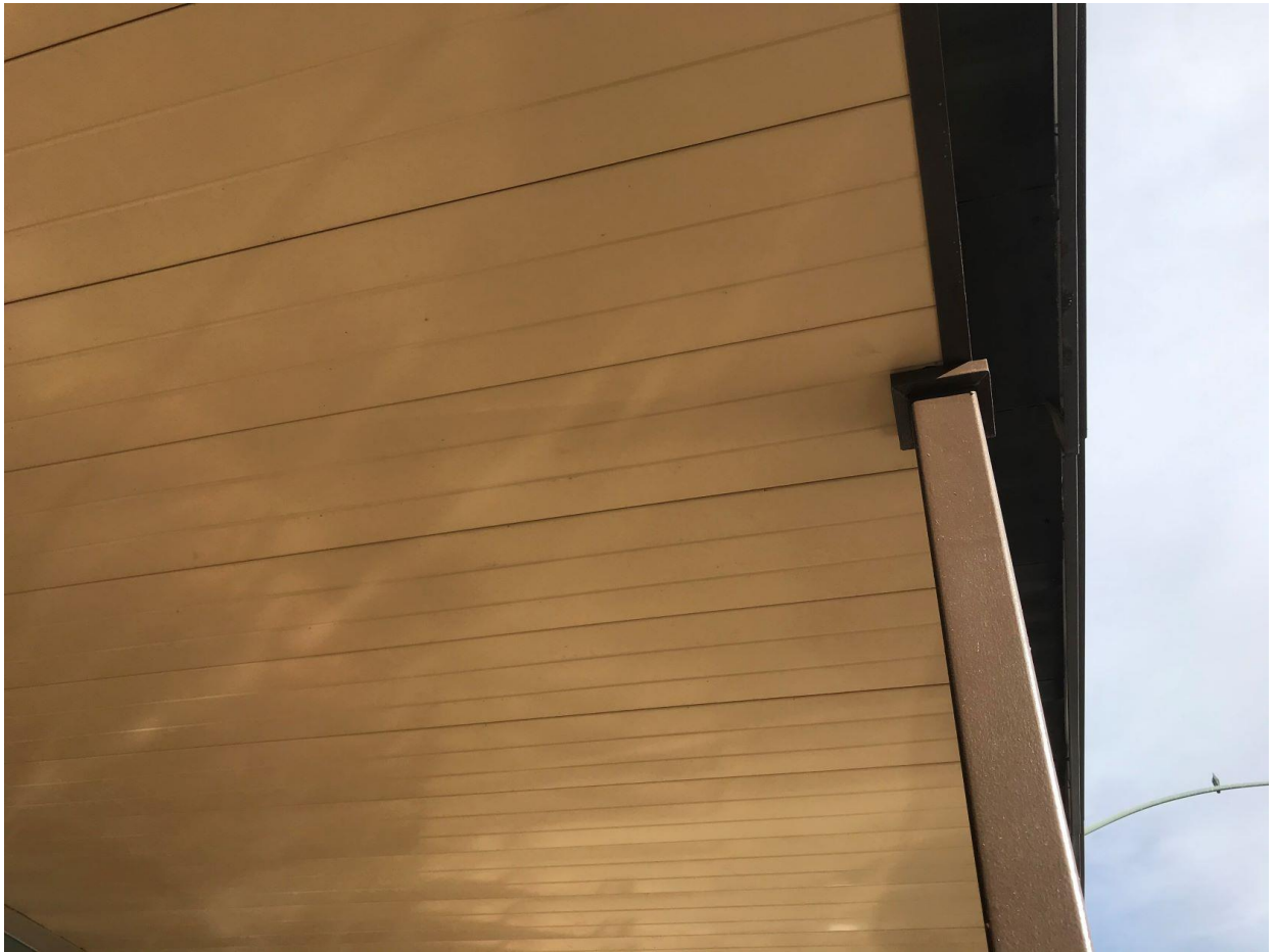
Detail of metal awning and supporting post. Cody's design originally had the post and beam meet in a flush configuration.
