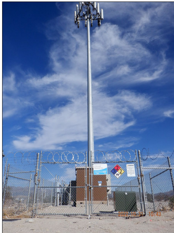
Figure 4. AT&T telecommunications facility.
