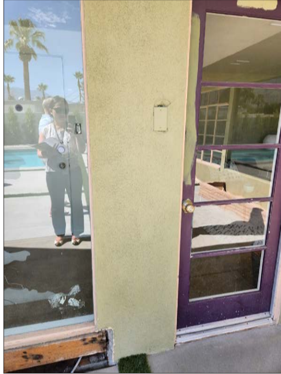
Image 9: Window and door removed for installation of sliding door (City of Palm Springs, 2023)
