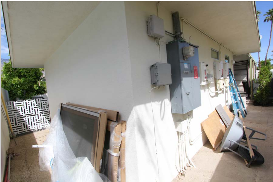
Image 50: South (left) and east (right) elevations of former maid's quarters, view northwest (Chattel, 2024)
