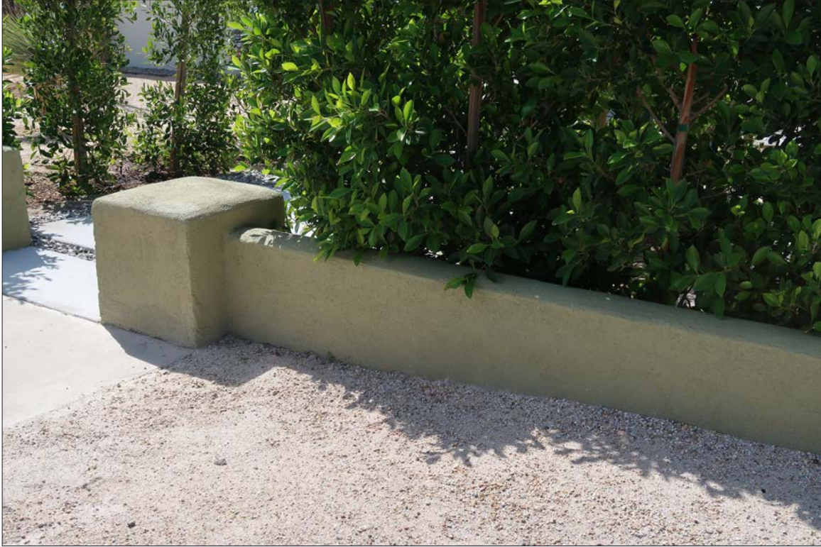
Image 23: Detail of low concrete wall at north of subject property, view southeast (Chattel, 2024)
