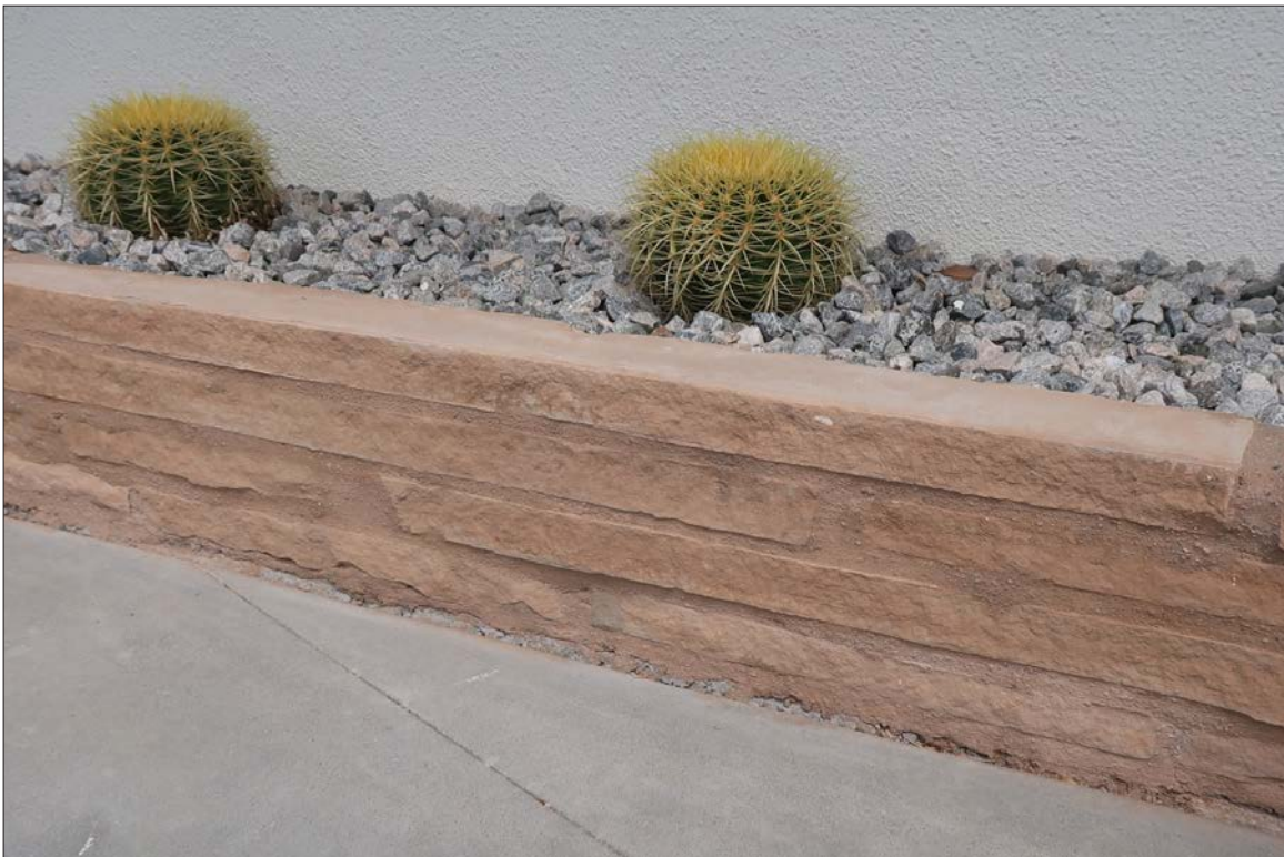
Image 44: Detail of mortar at south elevation planter (Chattel, 2024)
