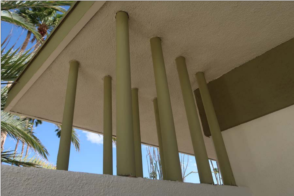
Image 31: Detail of vertical cylindrical poles where poles were cut to sit above added privacy wall, view northeast (Chattel, 2024)
