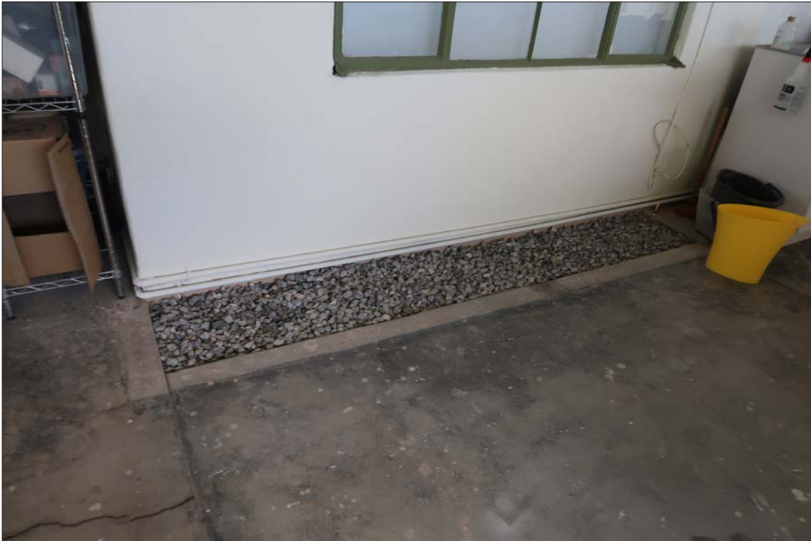
Image 57: Detail of area at east elevation where planter has been removed, view west (Chattel, 2024)
