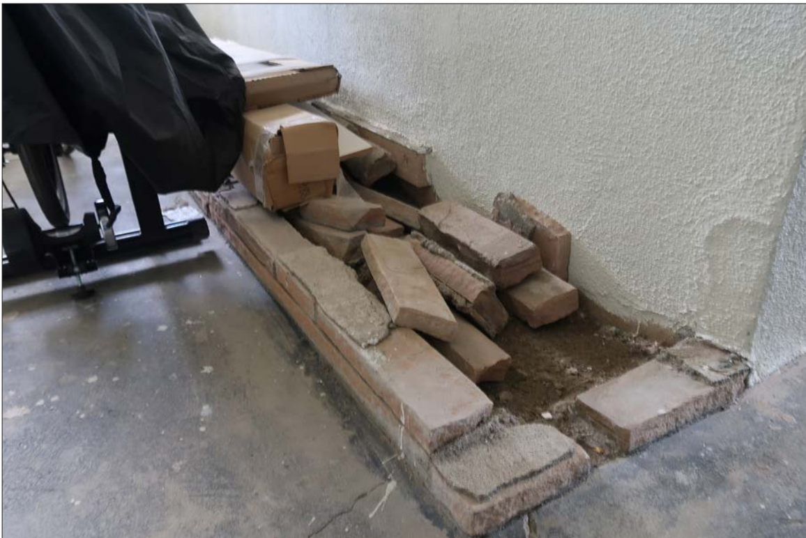
Image 58: Detail of demolished planter at north elevation of maid's quarters, view northeast (Chattel, 2024)
