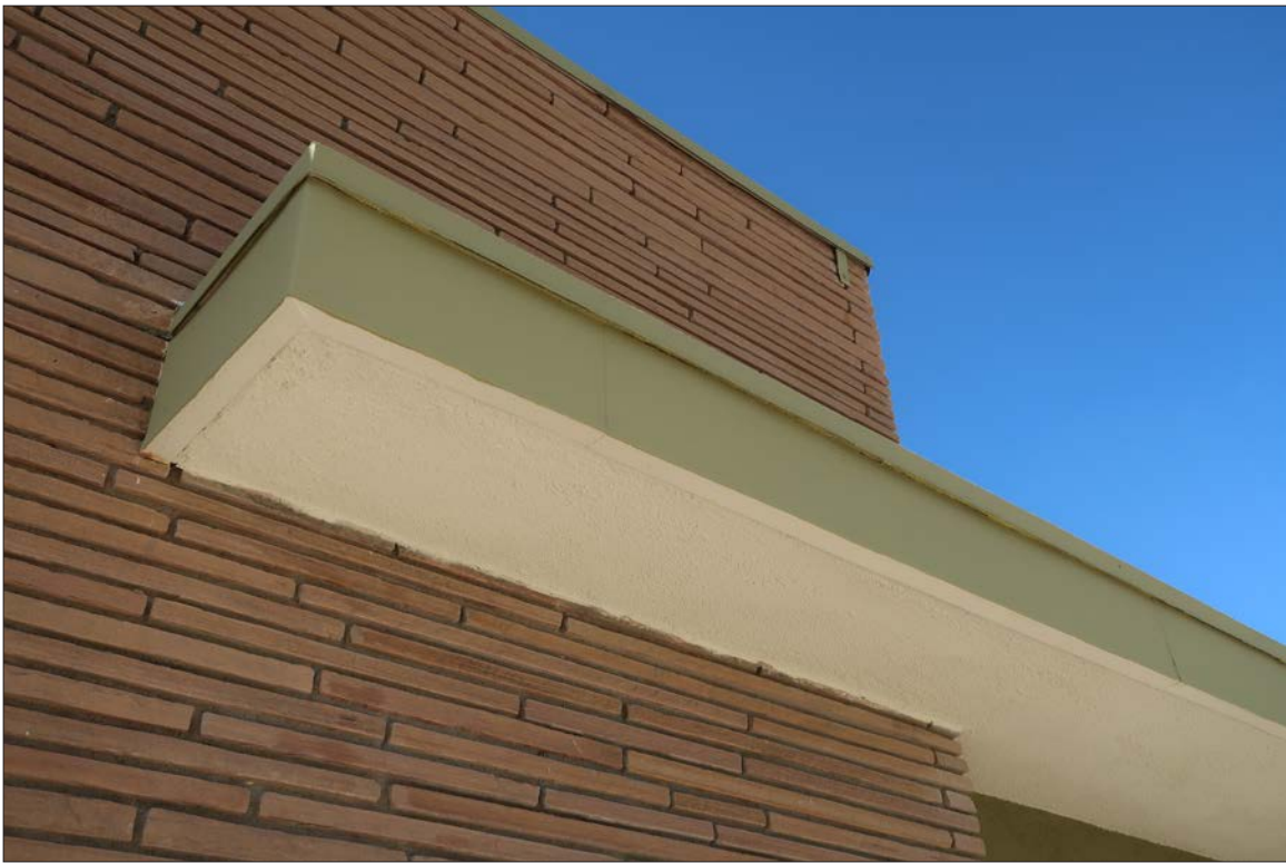
Image 20: Detail of eave continuing over chimney at north elevation, view southwest (Chattel, 2024)
