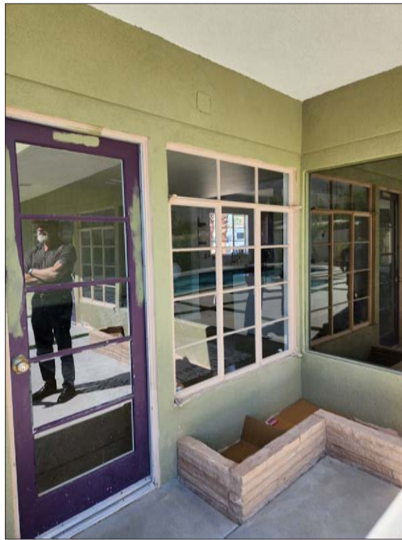
Image 10: Door removed for installation of south elevation sliding door at left (City of Palm Springs, 2023)
