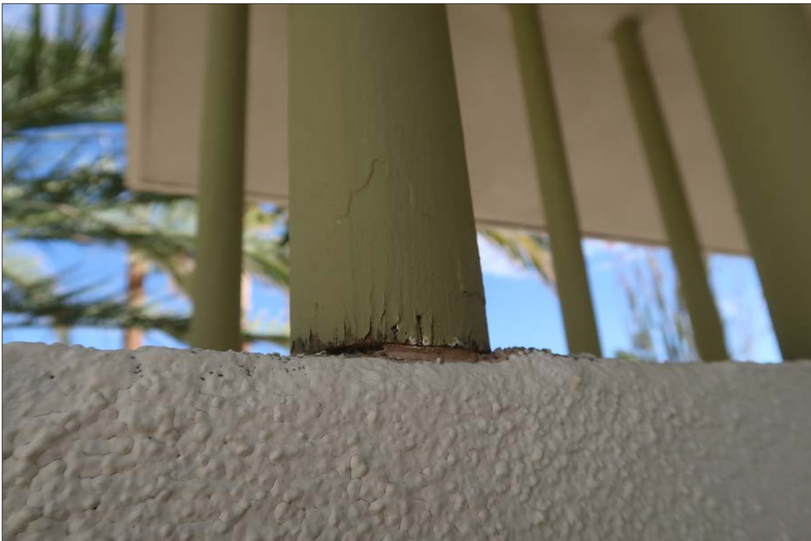
Image 32: Detail of vertical cylindrical pole showing wood material upon inspection, view northeast (Chattel, 2024)
